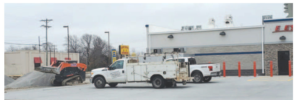
Work is nearing completion on a new Pete's convenience store on North Main in Miami.
