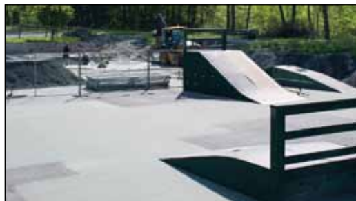
Old skatepark with wooden ramps in need of much repair
