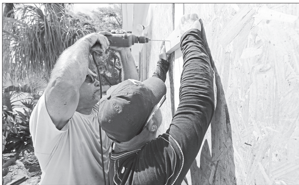
Peter Gonzalez and Jorge Abreu with Hurricane Busters Enterprises install hurricane shutters at a home in Key Largo in preparation for Hurricane Irma.
