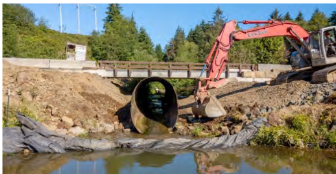
Peterson Creek bridge at the Miami River confluence during culvert removal in July 2020.
