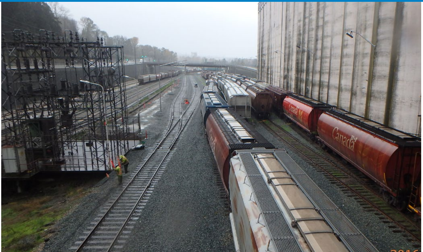
PNR RailWorks Pacific Region crews constructed these tracks and more for a large expansion project at the Cargill North Vancouver Rail Terminal.
