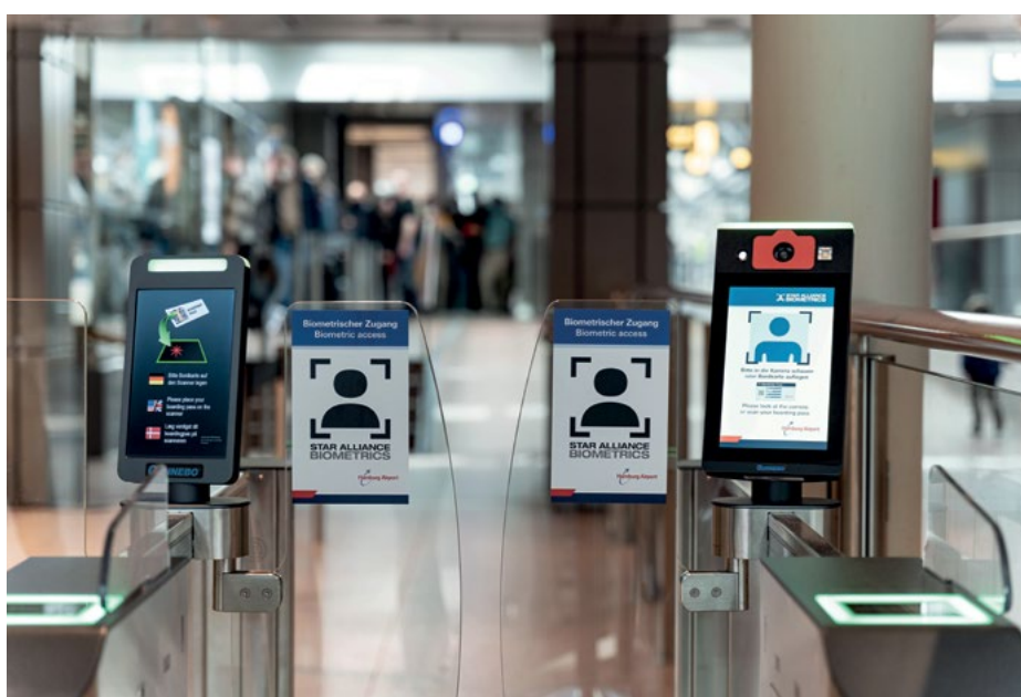
User-friendly: Star Alliance Biometrics installed at Hamburg Airport. Photo: Oliver Sorg
