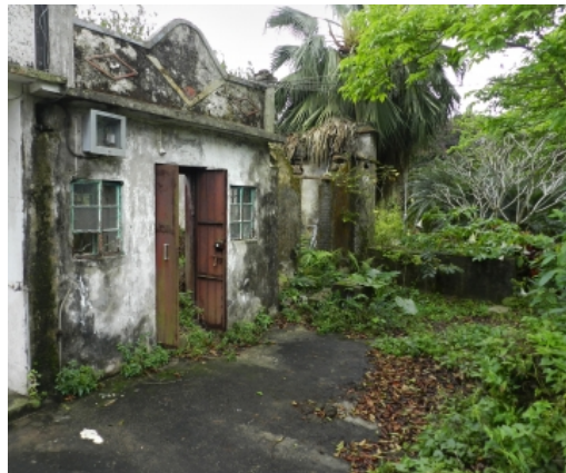
Some village houses like this one in the enclave village of Pak Sha O have been abandoned and begun to deteriorate over the years. Many landowners do not remodel the homes, instead choosing to sell the land to developers. Photo by Kelsey Tamborrino
