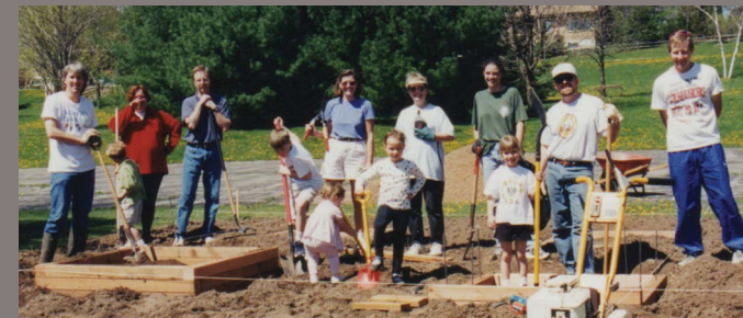
Parents, teachers, and students construct the first MCDS garden near the upper parking lot.
