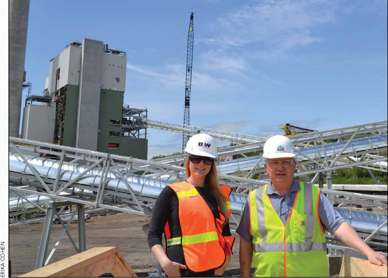
Alexandra Ritchie of Cate Street Capital and Site Manager Carl Belanger at the Burgess Biomass plant in Berlin.
