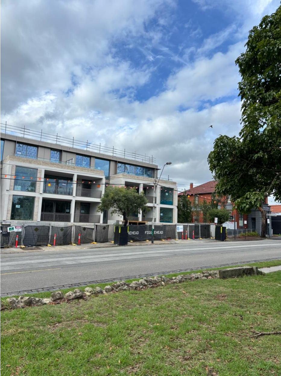
A four-storey apartment complex under construction next to liveability factors such as Central Park and the number 5 tram line on Wattletree Road in East Malvern.
