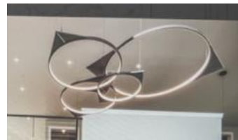
Hanging fixture in Great Room
