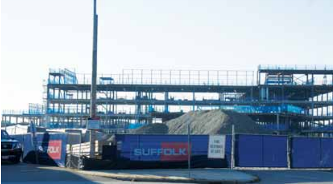
Though some workers could be observed, the Norwood Hospital site has seen at least a reduction in workers at the site in September.
