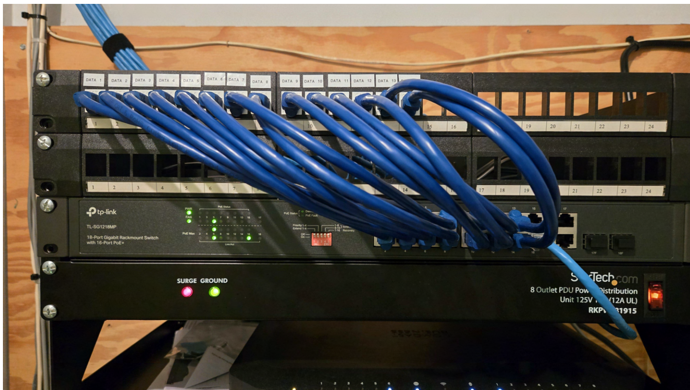
Completed rack-mounted network infrastructure with labeled patch-panel positions, managed switch, power distribution and business gateway.
