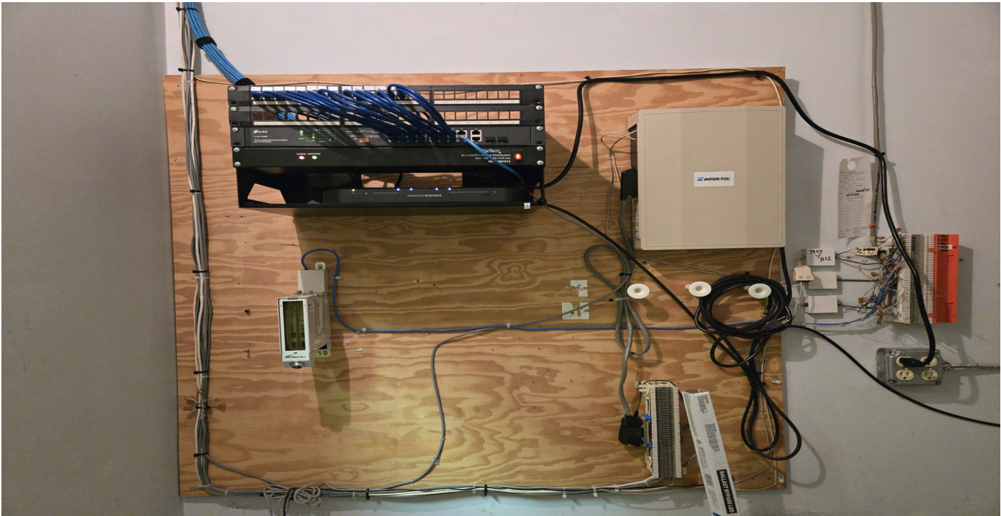
Final network area showing the completed rack installation and organized cable entry alongside existing communications infrastructure.
