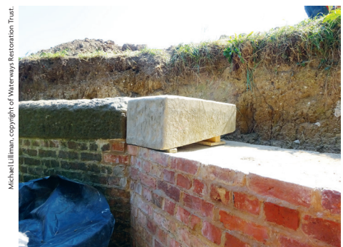
First new "stone" placed in position. The void at the back will be filled with lime mortar.
