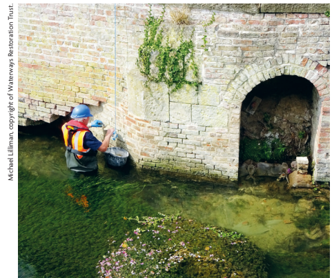
LNT member Pete repairing the arch support wall, working in waders. good job the weather was dry.
