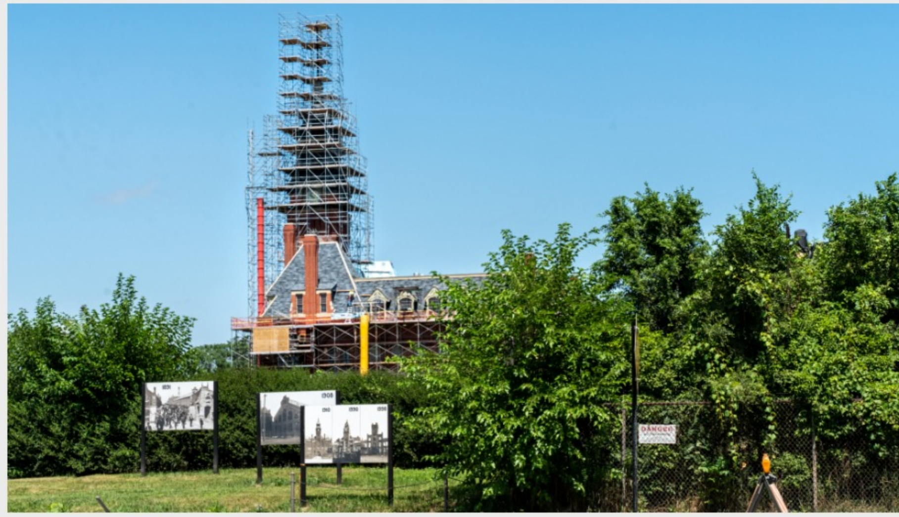
The Pullman National Monument, now undergoing extensive renovations, is comprised of the former administration headquarters of the Pullman Company.
