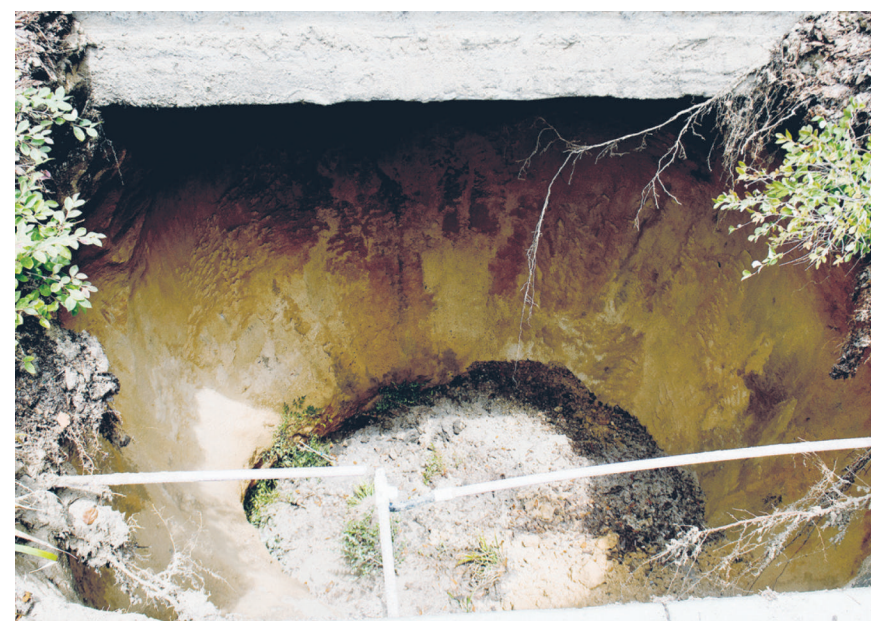
Sinkholes occur naturally in this part of the country, often after periods of significant rainfall.
