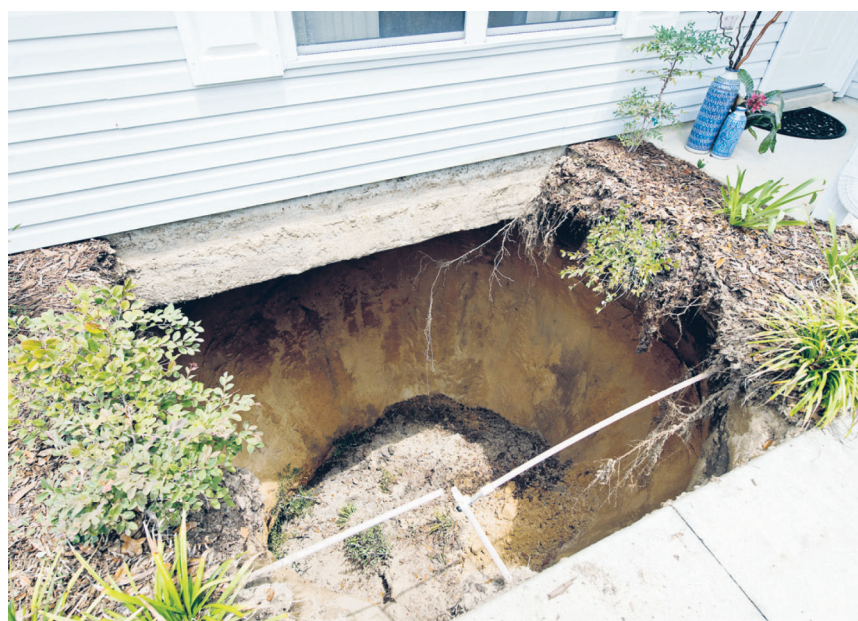
A Villager in the Village of Liberty Park awoke Saturday morning to find a roughly fifty foot deep sinkhole had formed under the front portion of her home.
