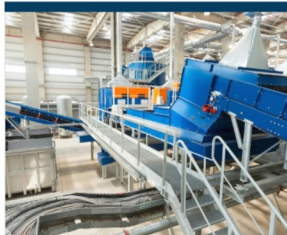
Waste to Energy Plants
