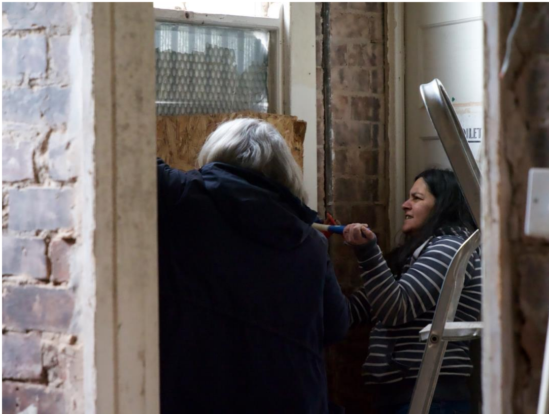
Brown's friend Debbie Ramsdale is passing her a drill to remove a curtain track. She also helps Brown to remove a soaked wooden cover of a window.
