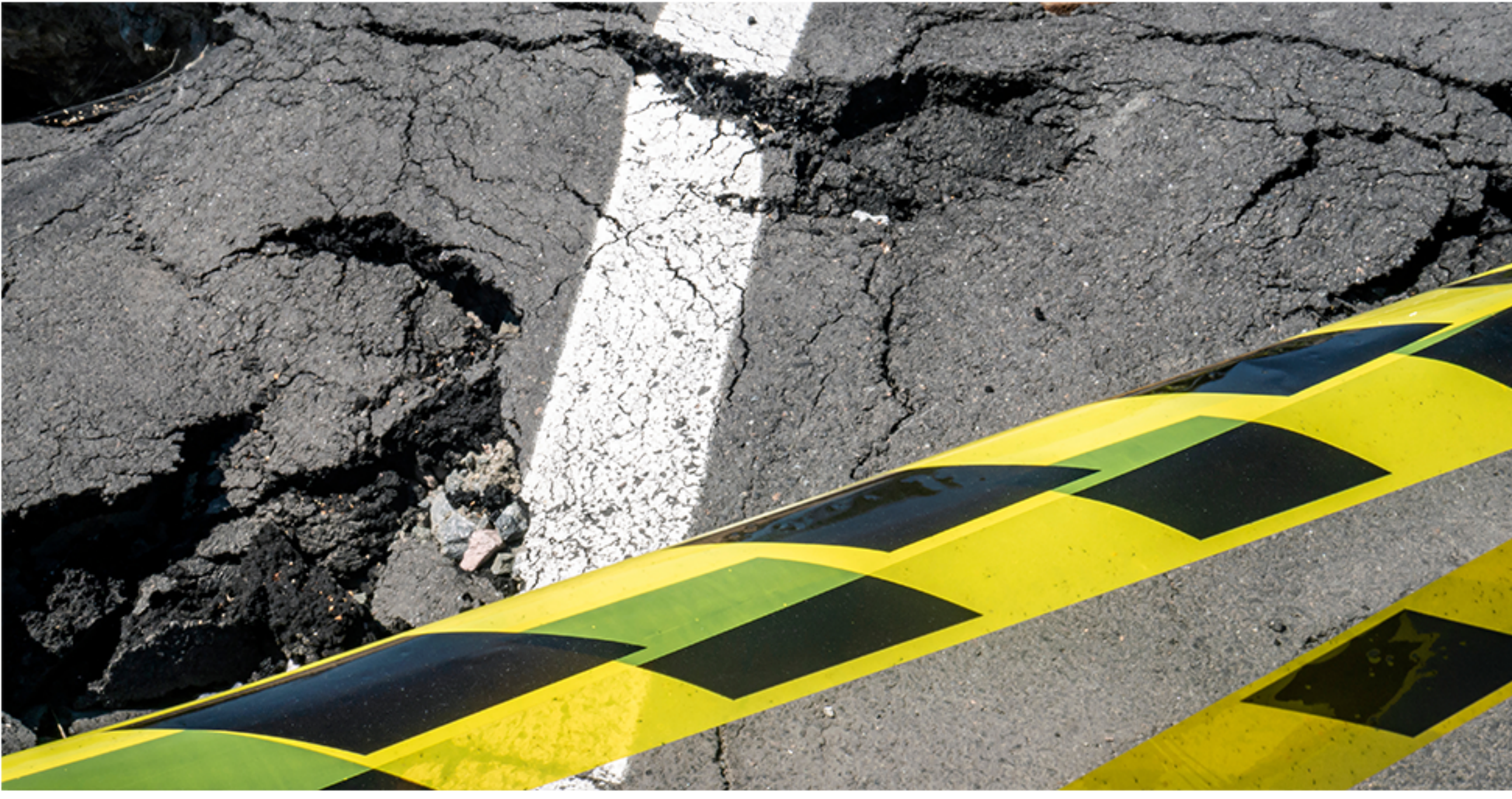
Part of the road in Garforth had started to crumble following the underground water main burst
