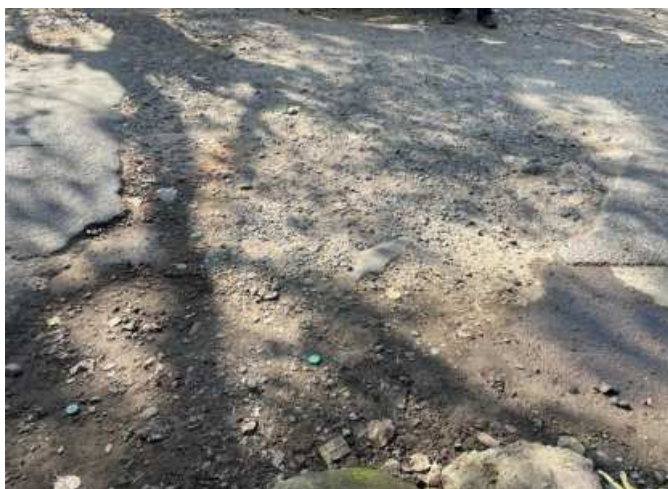
Kathivakkam High Road; and the space below the flyover. PHOTOS : SPECIAL ARRANGEMENT
