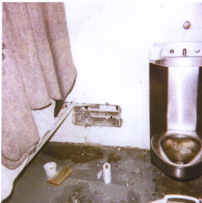
A leaky toilet and hole in vent are illustrations of poor conditions at the Blackfeet jail. Photo courtesy of Blackfeet Law Enforcement Services
