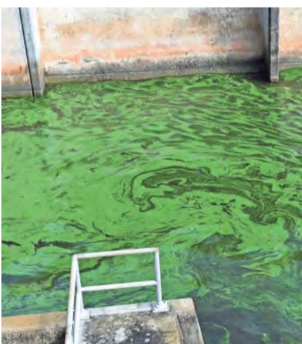
Algae and water condition seen around the St. Lucie Lock and Dam along the C-44 canal Monday in Martin County. The Army Corps of Engineers suspended discharges of Lake Okeechobee algae-filled water again late Sunday. ERIC HASERT/TCPALM
