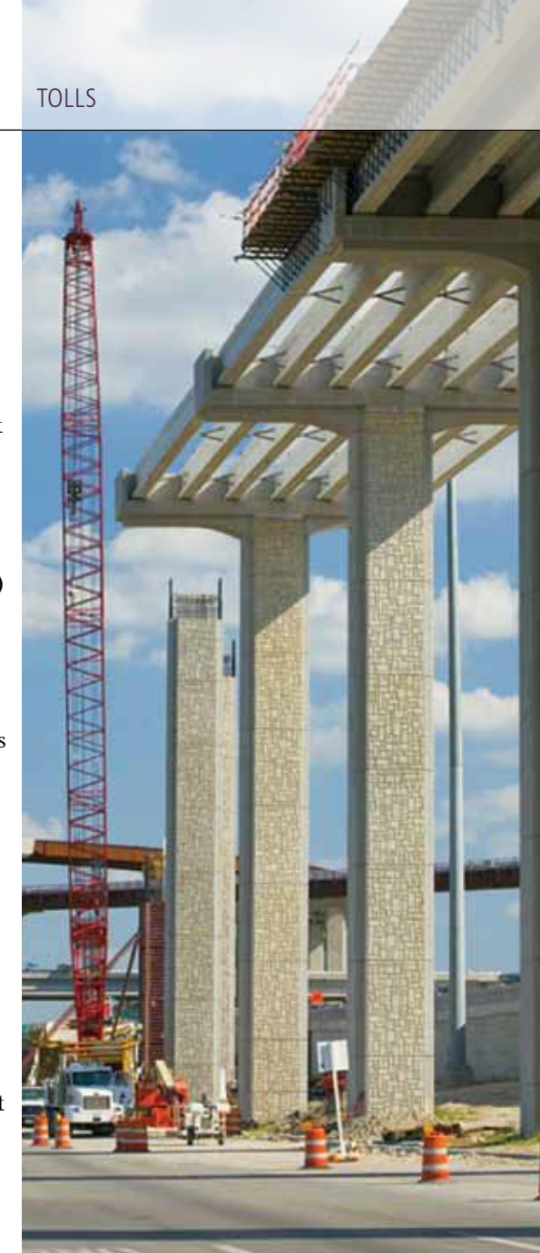
As part of TxDOT's $3.6-billion CTTP, PBS&J managed construction of the SH 45 & US 183 direct connector.
