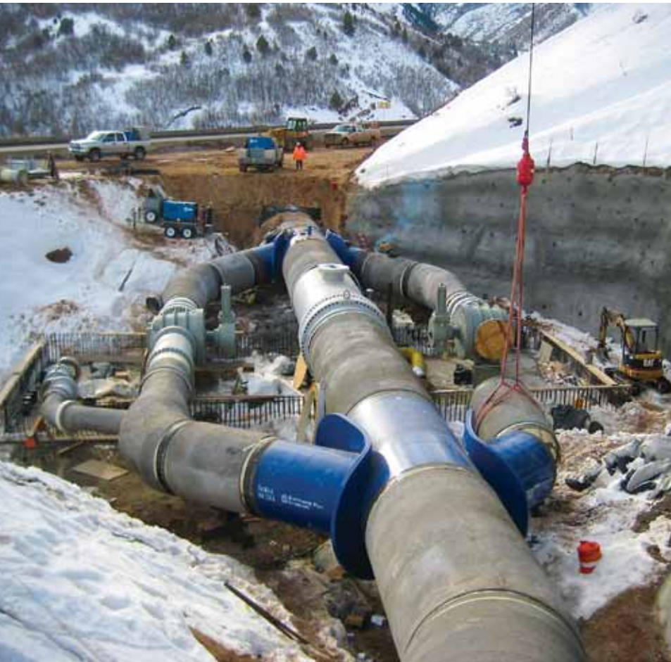
Metering station for mortar-coated steel pipe.
