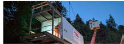
ABB ensures power in Swiss tunnels
