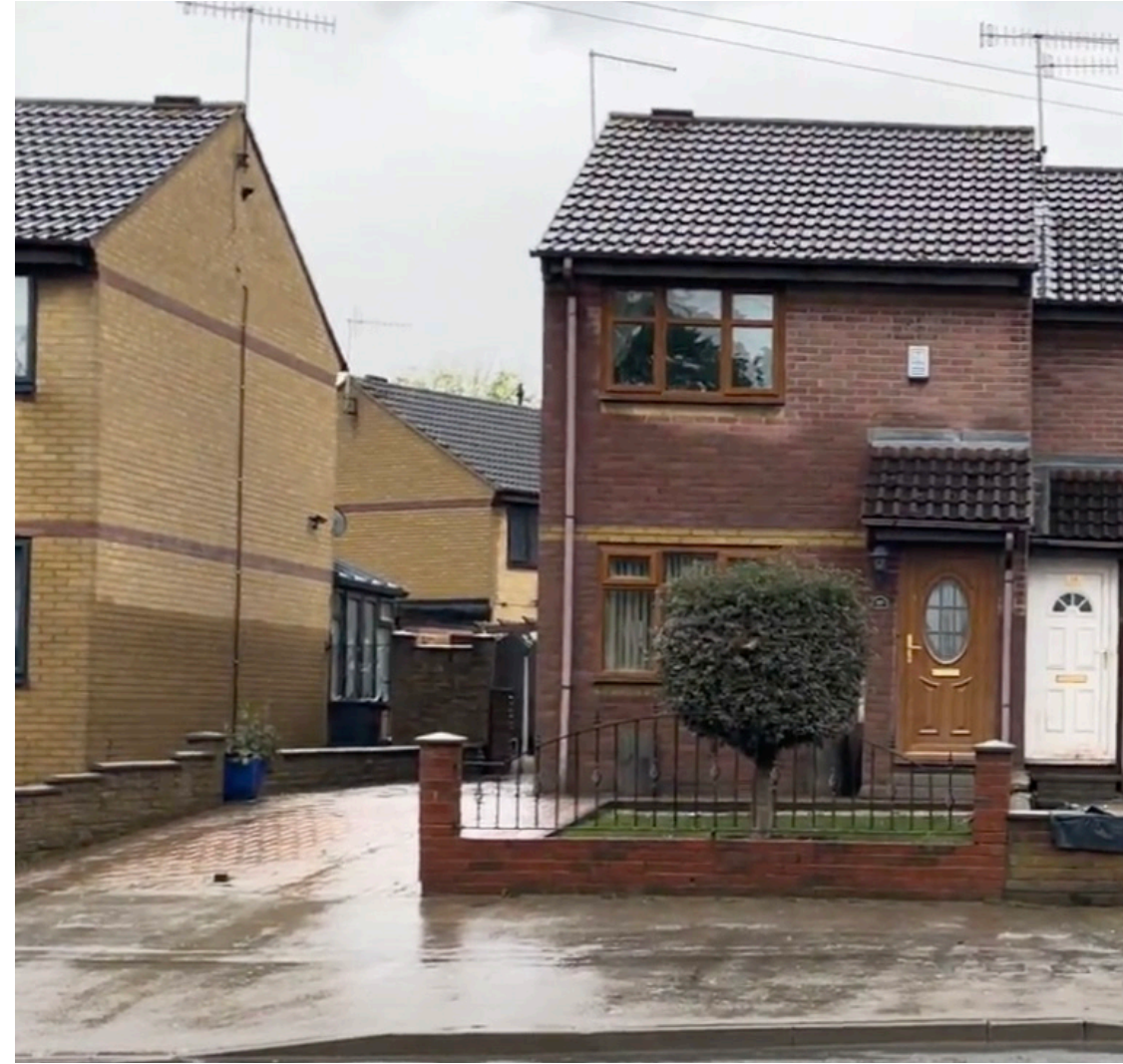
Damp patches on the bricks indicating
