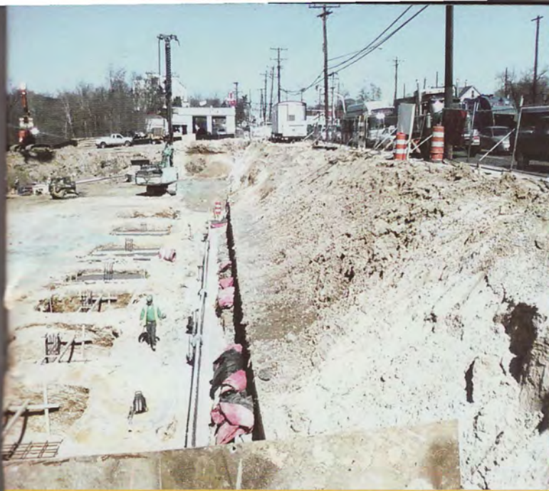
After the Impact System is installed, crews prepare to pour spread footings.
