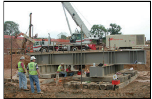
Load testing of the micropile support system at New Design Road Water Treatment Plant in Frederick, Md.
