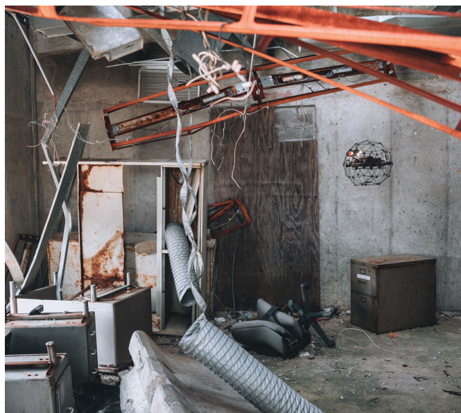
◀ Drones mitigate the need for enclosed-space entries by maintenance personnel, which is helping to improve safety in industrial facilities. They can help personnel inspect damaged or malfunctioning structures without putting humans at risk, and can help companies save millions of dollars. Image courtesy of Flyability.
