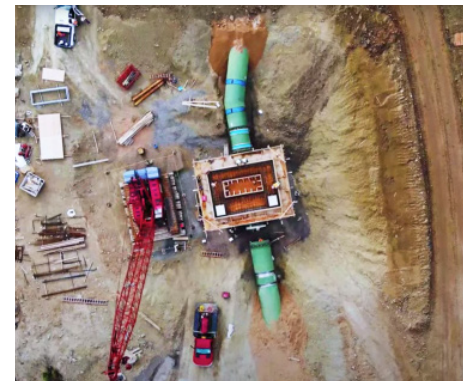
Northwater Treatment Plant in Denver, Colorado
