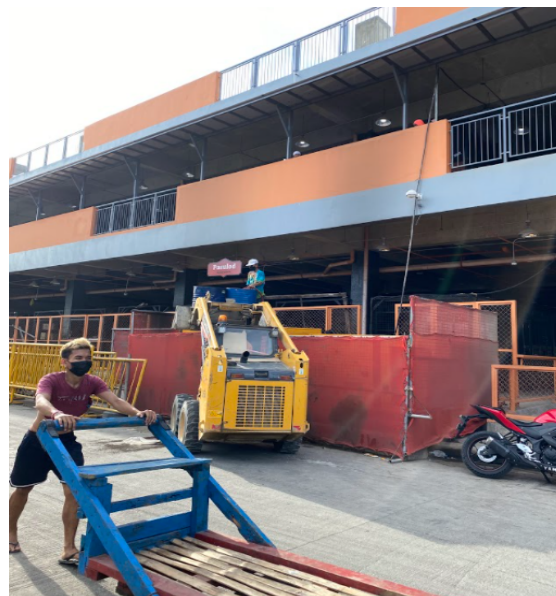
Boy pushes a cart in front of the new Carbon Market under construction
