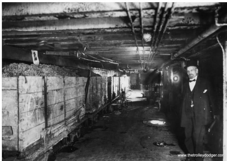
An ash car train in the Marshall Field and Company boiler room on February 16, 1915. Picture by thetrolleydodger
