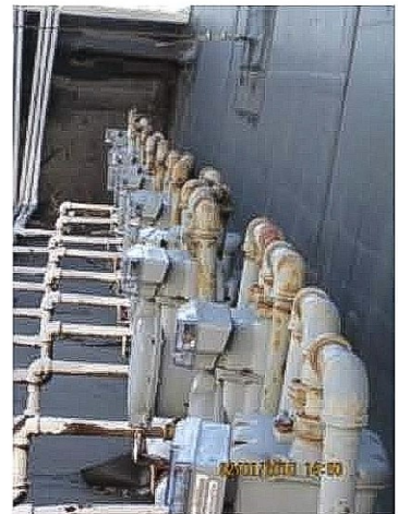
Electricity meters at the Cameron Butcher building in downtown Colorado Springs. Cameron Butcher, a commercial real estate group, is one of 12 businesses participating in the audit program to determine how to use resources efficiently.
