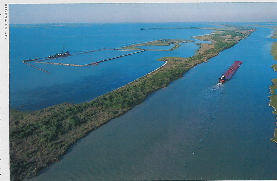
Bird Islands: One finished (top center), one under construction (adjoining on left).
