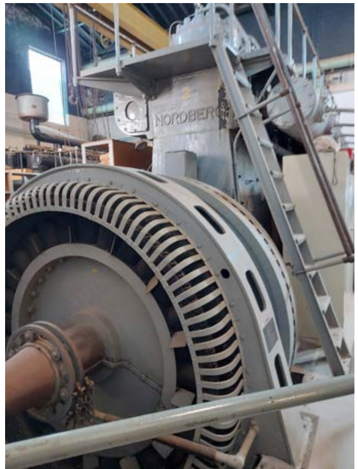
Outdated generator in existing City of Sioux Falls power building
