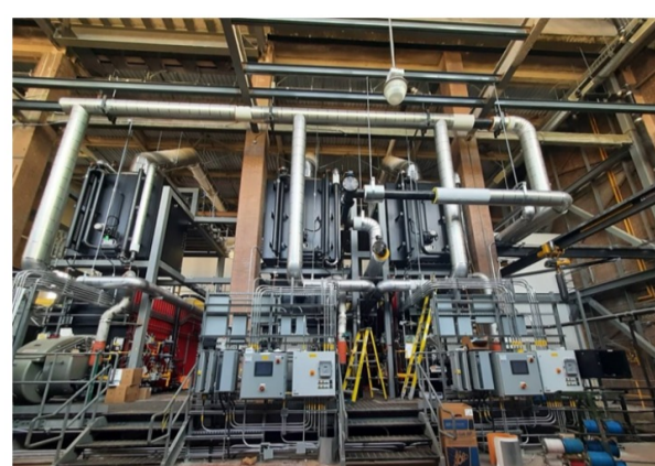
New boiler plant at Confederation Heights
