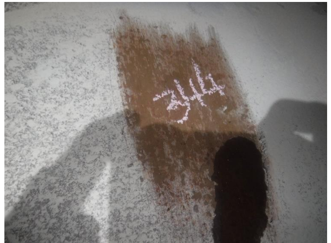
INT 26 – 20'± – Oxidation present behind buildup
