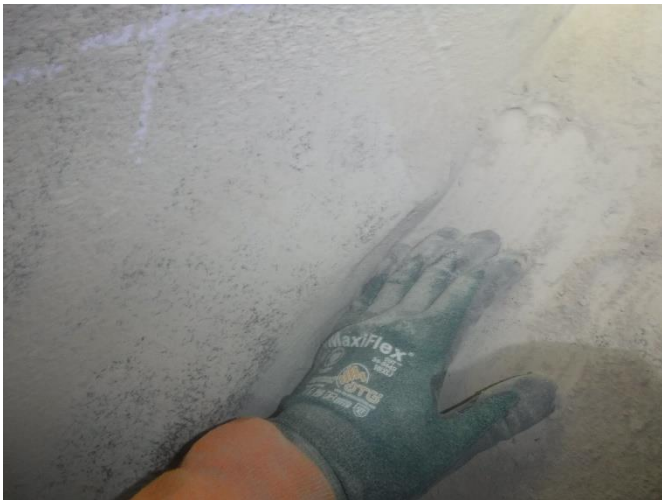
INT 13 – Buckling in the corner of duct
