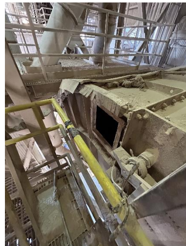
EXT 10 – Access door to the duct
