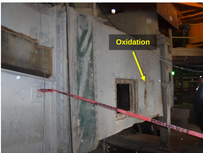
EXT 21 – Side of the east pant leg; oxidation on access door
