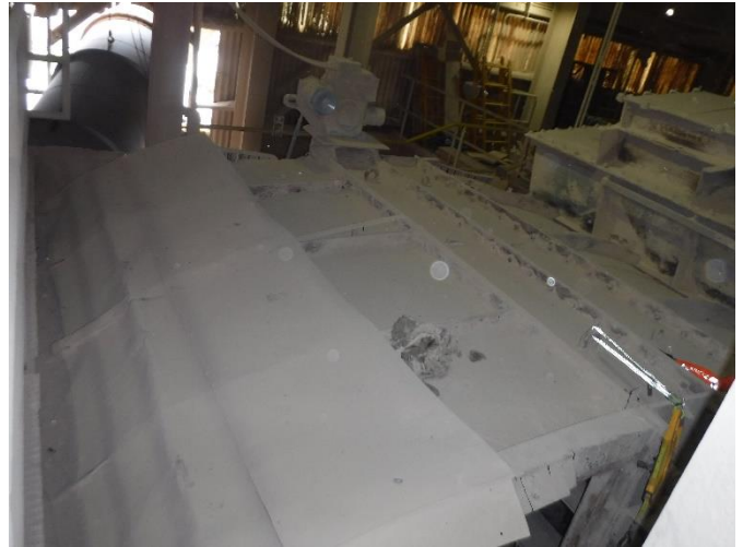
EXT 18 – Debris and buildup on duct
