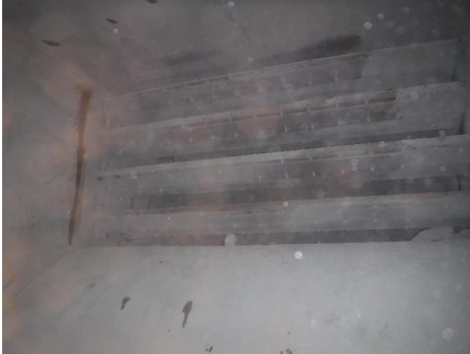
INT 11 – Buildup on damper blades
