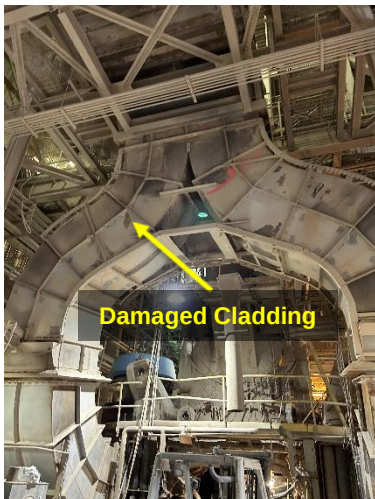
EXT 9 – Damaged cladding
