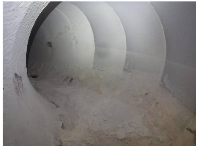
INT 32 – Heavy buildup and debris
