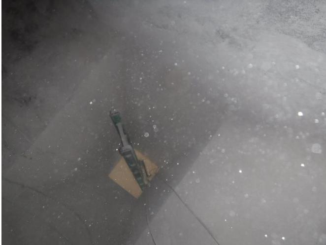
INT 29 – Ladder in the opening below the duct
