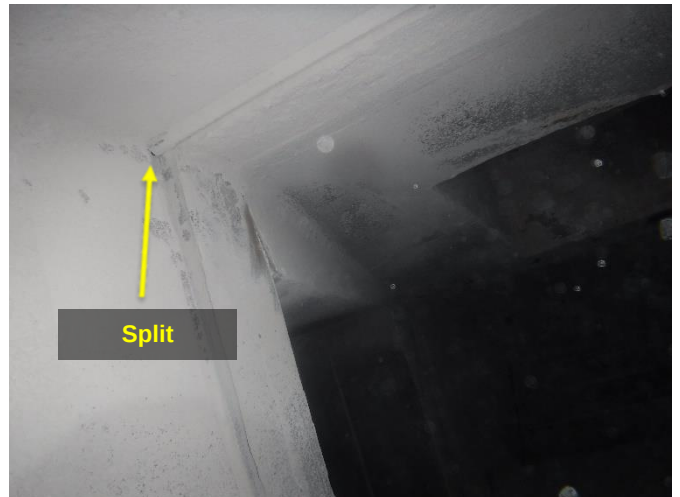
INT 28 – 16'± – The top West side of the duct is split
