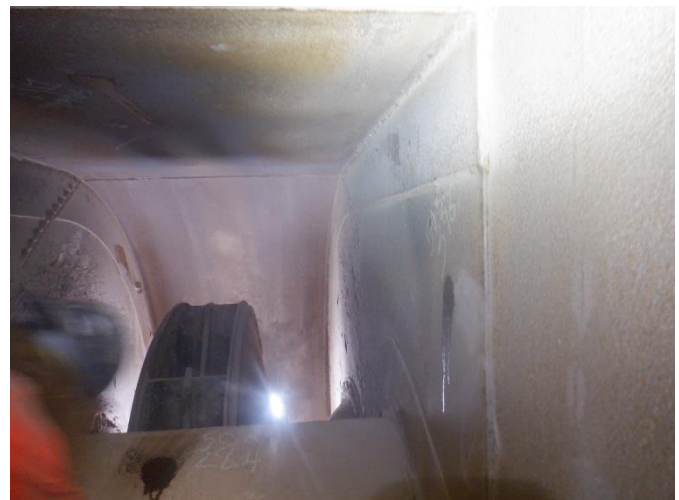
INT 40 – Duct curling downward
