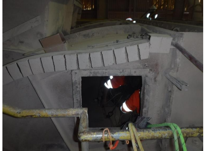
EXT 12 – Access door to the duct
