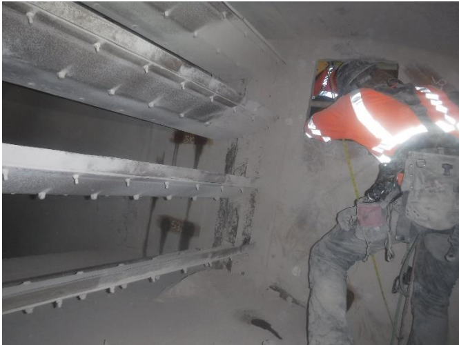
INT 7 – Buildup on damper blades
