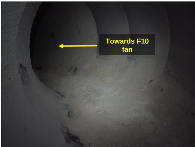
INT 31 – Looking forward towards f10 fan
