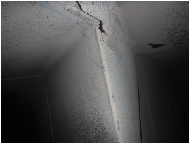
INT 21 – 11'± – The metal panel is torn on the floor of the West side
