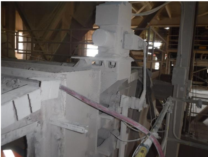
EXT 13 – Light buildup on top of duct
