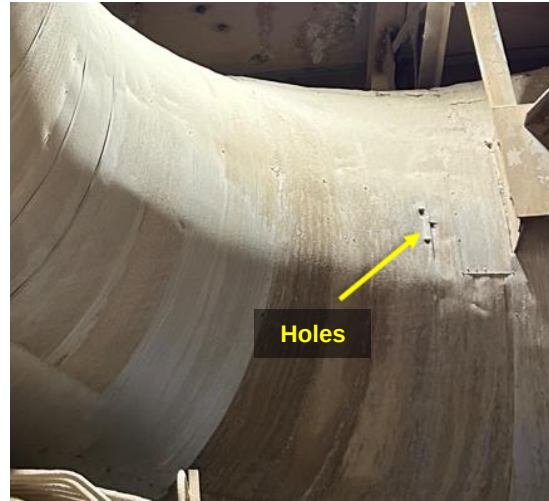
EXT 6 – Holes in the duct
