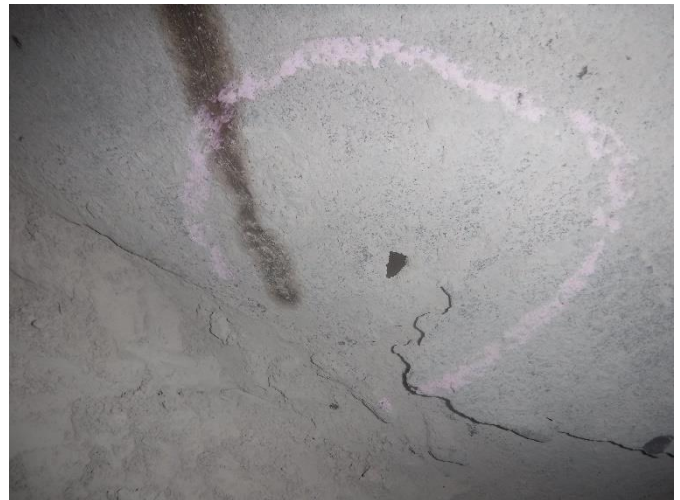
INT 14 – 13"± – 0.5" hole present in the east side of the duct
