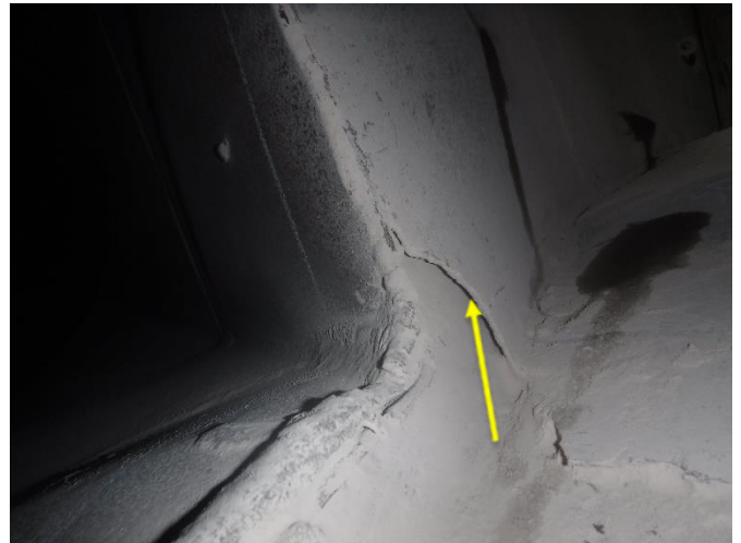
INT 20 – 11'± – The metal panel is torn on the floor of the West side
