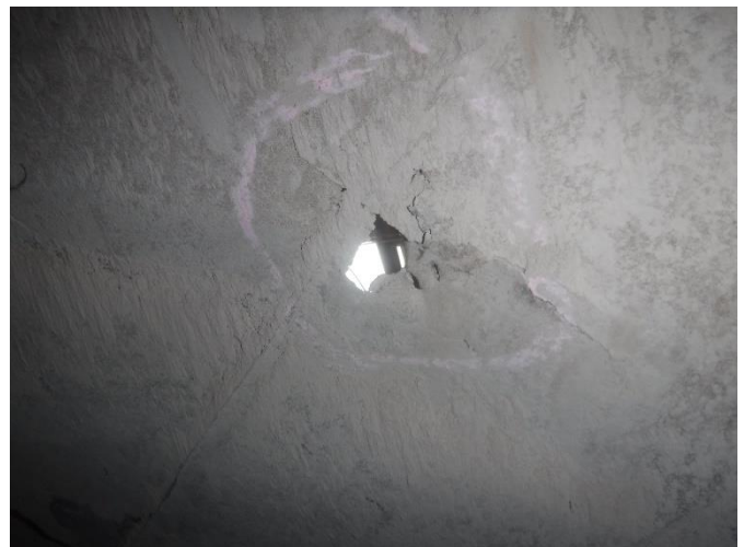
INT 16 – 13"± – 1.5" hole present in the east side of the duct
