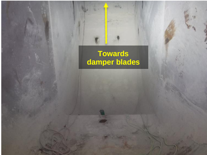
INT 35 – Looking back towards damper blades
