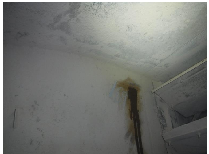
INT 10 – Corner of damper blades
