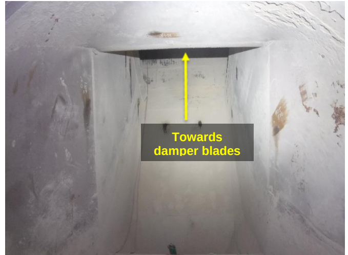
INT 36 – Looking back towards damper blades
