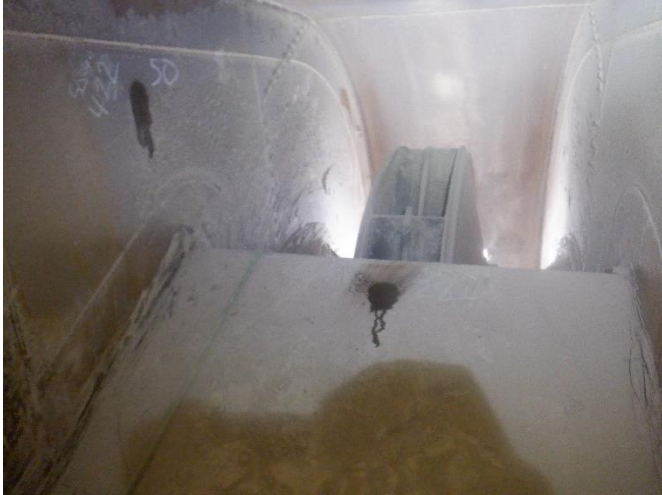
INT 41 – Duct curling down outside of the building going to fan
