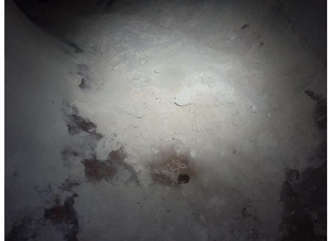
INT 30 – Looking forward duct; Debris and buildup present on duct floor
