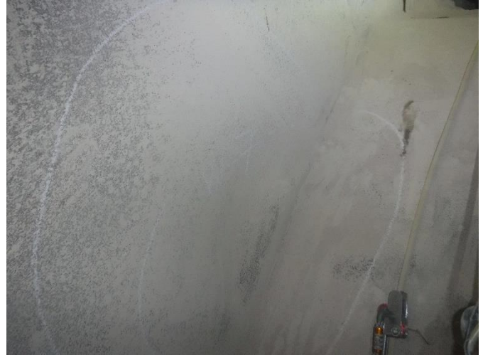
INT 12 – Buckling in the corner of duct
