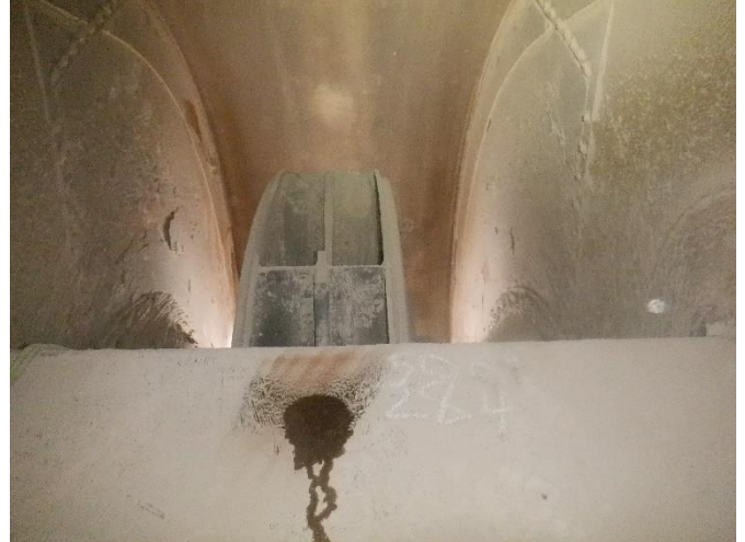
INT 42 – Duct curling down outside of the building going to fan
