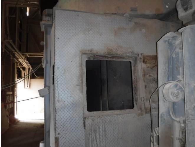
EXT 23 – Oxidation on the access door at the end of the east pant leg
