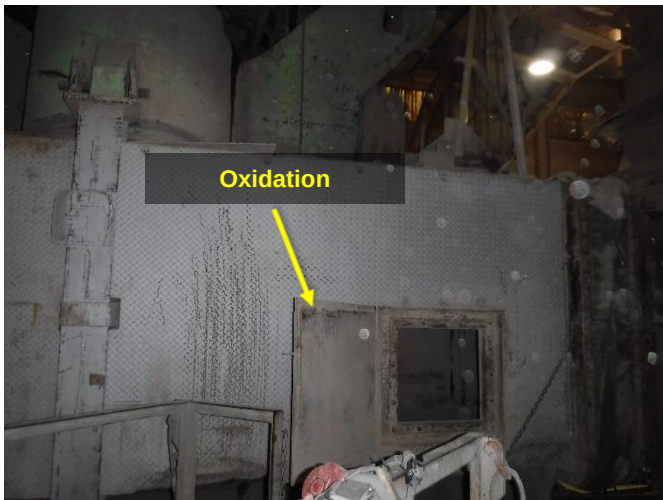
EXT 25 – Oxidation on the access door on the west pant leg
