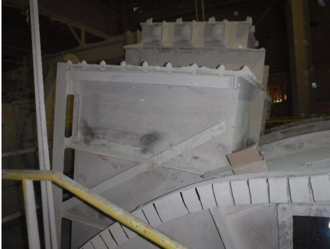
EXT 11 – Light buildup on top of duct
