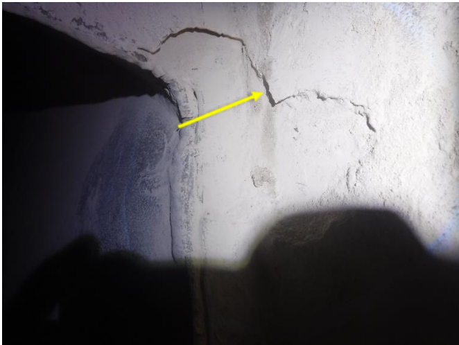
INT 19 – 11'± – The metal panel is torn on the floor of the West side
