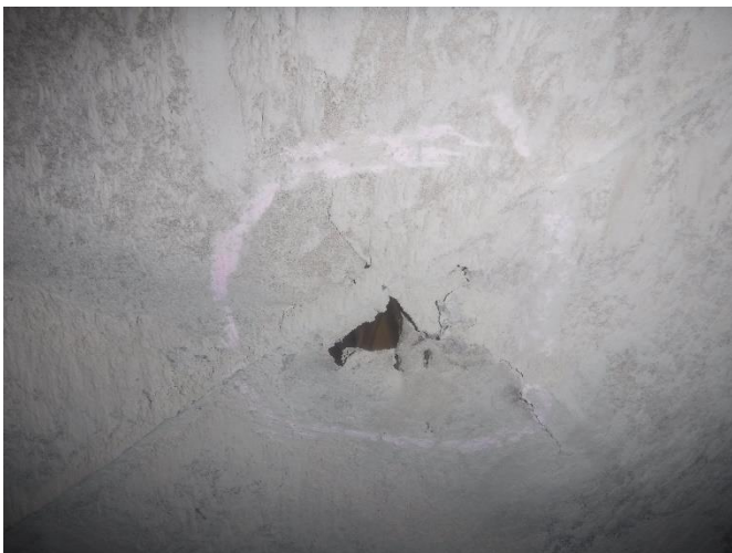
INT 15 – 13"± – 1.5" hole present in the east side of the duct
