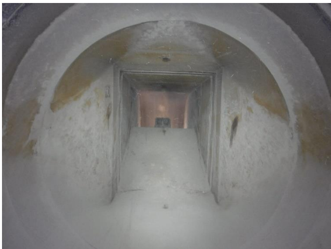
INT 39 – Duct curling downward
