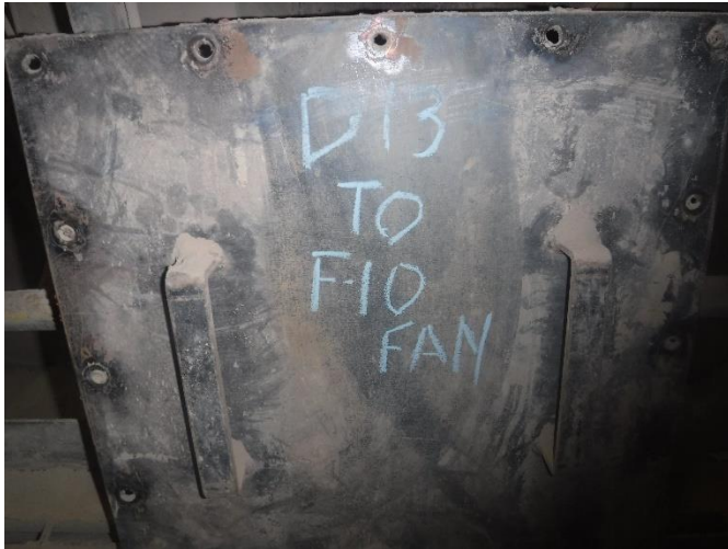
INT 1 – Access door leading to F10 fan
