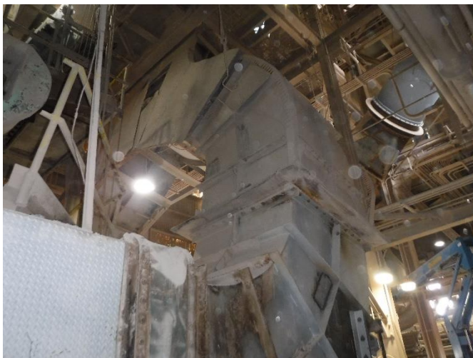
EXT 27 – Oxidation present on vent
