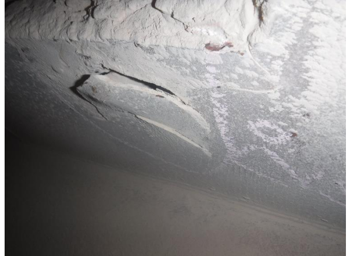
INT 24 – 16'± – The ceiling of the duct is damaged
