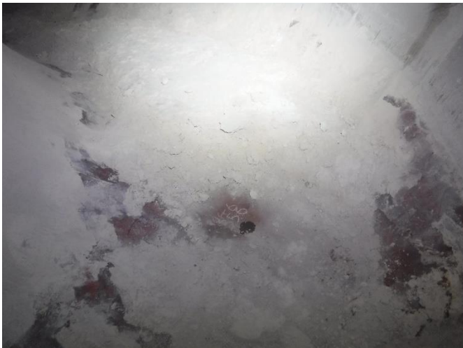
INT 33 – Heavy buildup and debris
