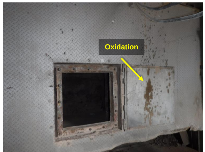
EXT 22 – Oxidation on door
