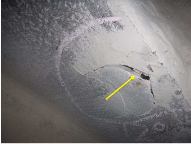
INT 23 – 16'± – The ceiling of the duct is damaged
