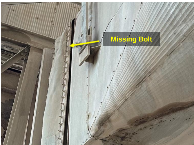
EXT 3 – Missing bolt on expansion joint
