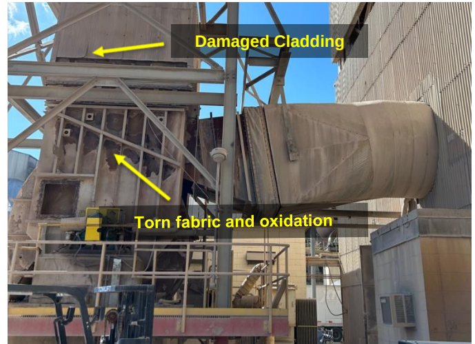
EXT 2 – Oxidation present behind torn fabric and damaged cladding
