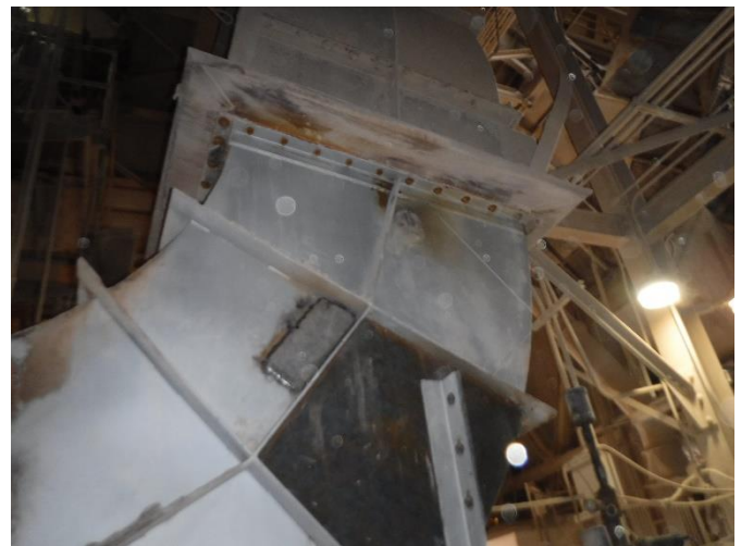
EXT 28 – Mild to severe oxidation on the side of the west pant
