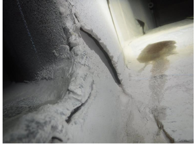
INT 18 – 11'± – The metal panel is torn on the floor of the West side
