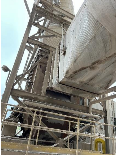
EXT 1 – Buildup on the outside sections of duct; oxidation on expansion joint.
