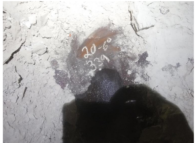
INT 38 – Heavy debris and buildup
