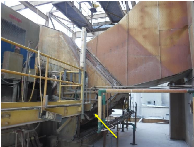
EXT 43 – Breeching showing oxidation and damaged cladding
