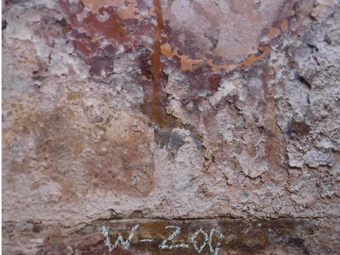
INT 5 – EL. 213'± – Buildup and oxidation present on surface
