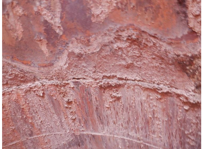
INT 6 – EL. 190'± – Buildup on steel plates
