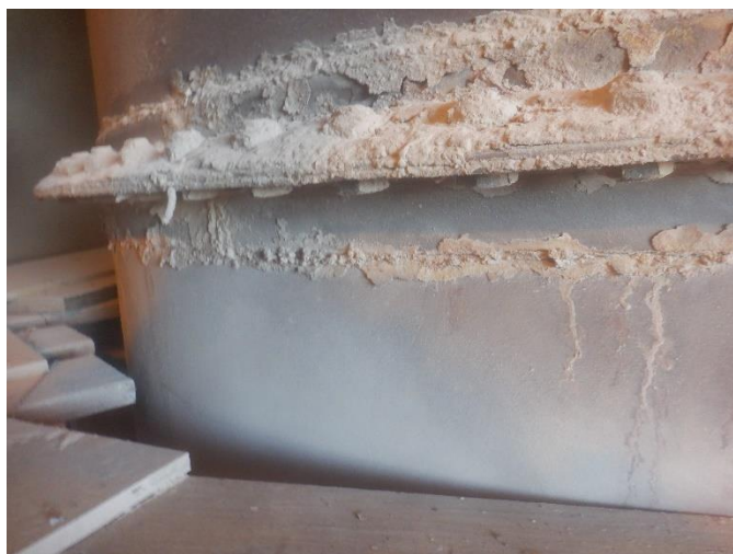
IMG 25 – View of hole with buildup present (caused by flue leakage)
