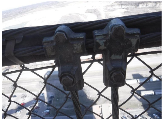
EXT 16 – Roof – Conductors connected to the building's LPS
