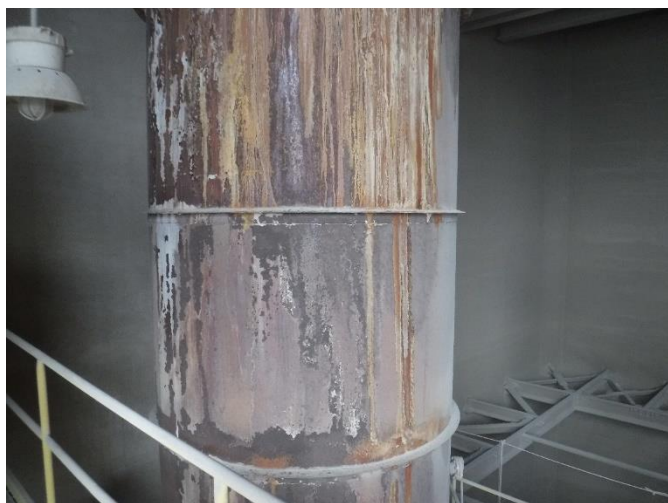
EXT 21 – 10 th floor – Stack showing oxidation and stains from leaking
