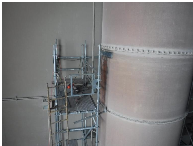
EXT 33 – 7 th Floor – Leakage stains from cracked flanged joint; scaffolding and repairs in progress
