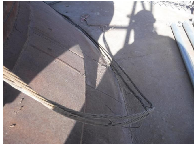
EXT 14 – Roof – Frayed LPS conductor
