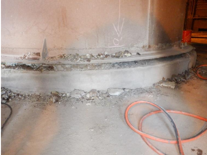
IMG 9 – The base before repair process
