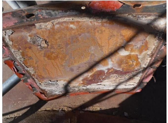
EXT 6 – Oxidation on the backside of the access door
