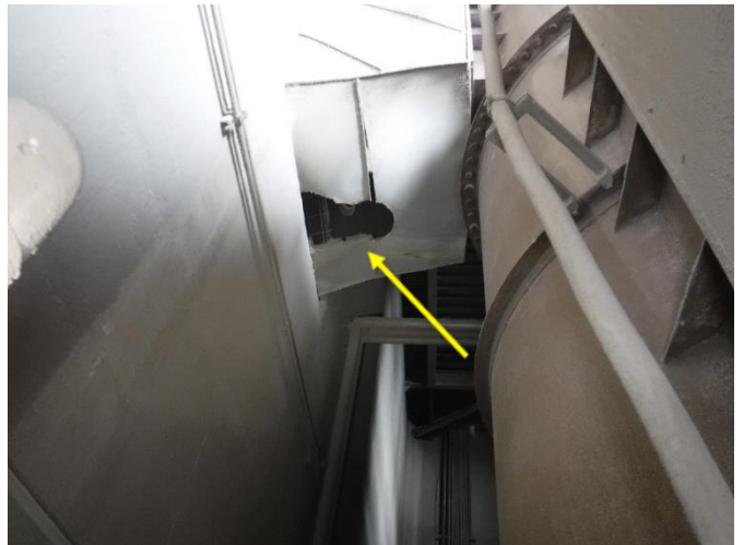
EXT 40 – View of duct with perforation on the bottom
