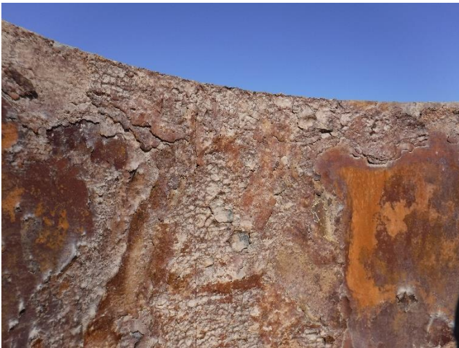
INT 3 – EL. 213'± – Top of the stack, buildup heavy oxidation
