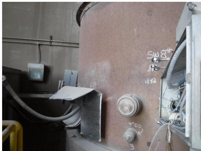
EXT 30 – Exposed wiring on instrument
