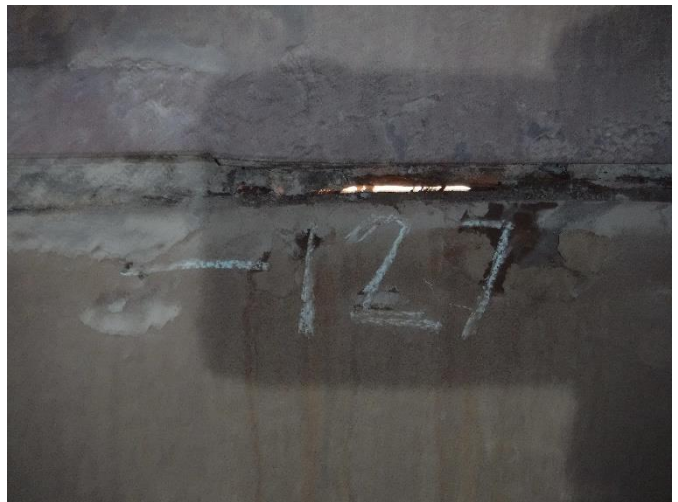
INT 28 – W EL. 127'± – Gap in flanged joint
