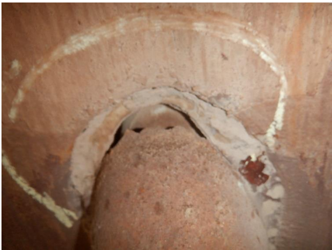
INT 27 – E EL. 140'± – Corrosion hole present in instrument port nozzle
