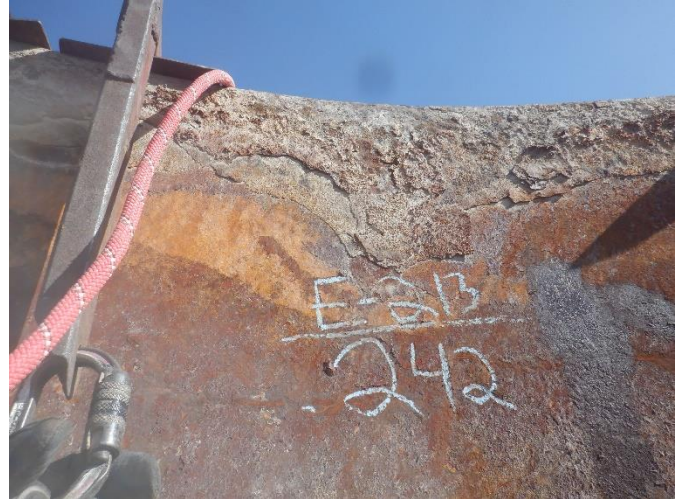
INT 2 – EL. 213'± – Top of the stack, buildup heavy oxidation
