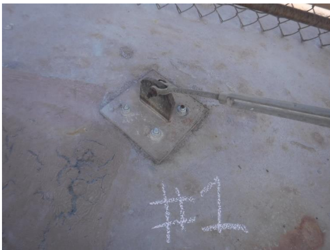
EXT 9 – Guy wire anchor
