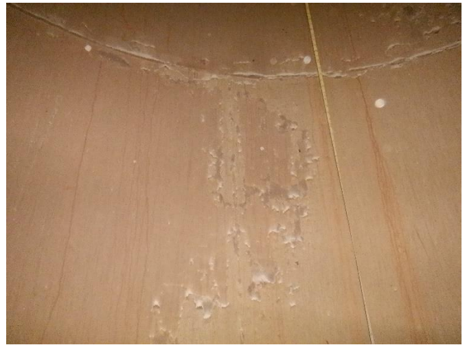
INT 38 – E EL. 90± – Upward view of weld joint and buildup
