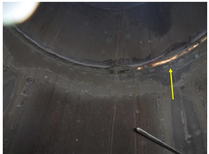
INT 32 –W EL. 115'± – Upward view of stack; gap in flanged joint
