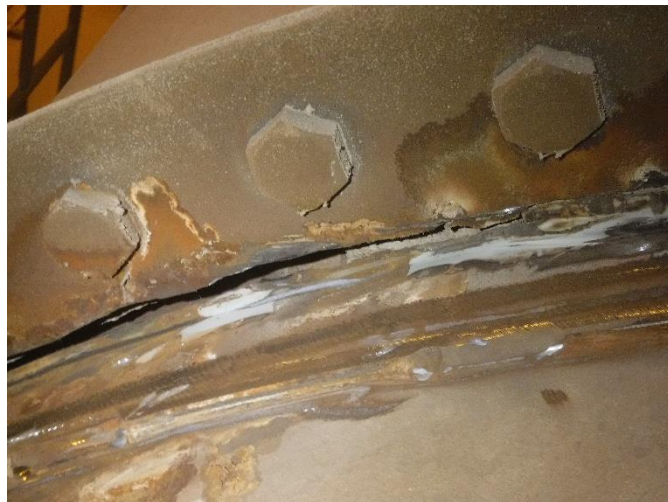
IMG 34 – Closeup of cracked weld
