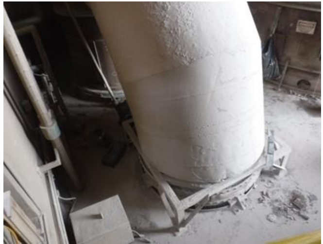
EXT 42 – 6 th floor – Expansion joint and Breeching duct with mild debris on floor
