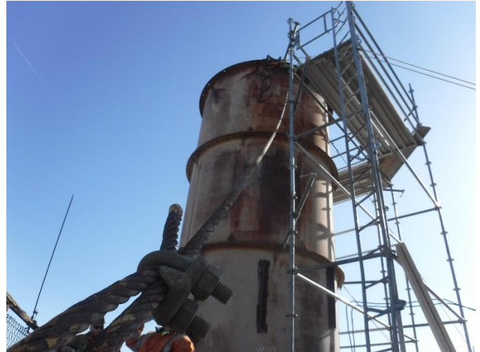
EXT 2 – View of the stack above the roof. Heavy oxidation present.
