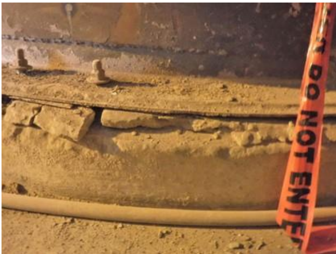
IMG 15 – The base before repair process
