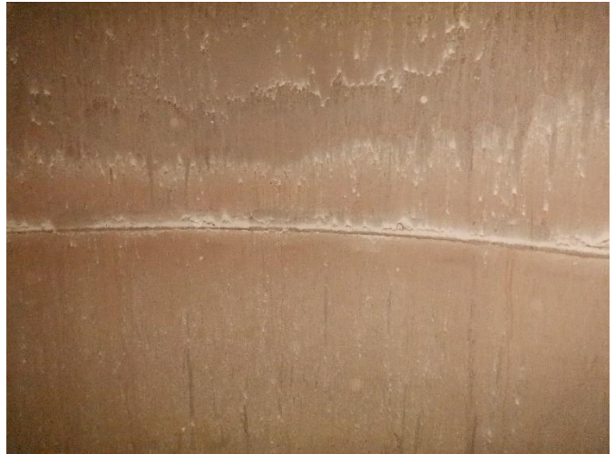
INT 24 – E EL. 140'± – View of flanged joint
