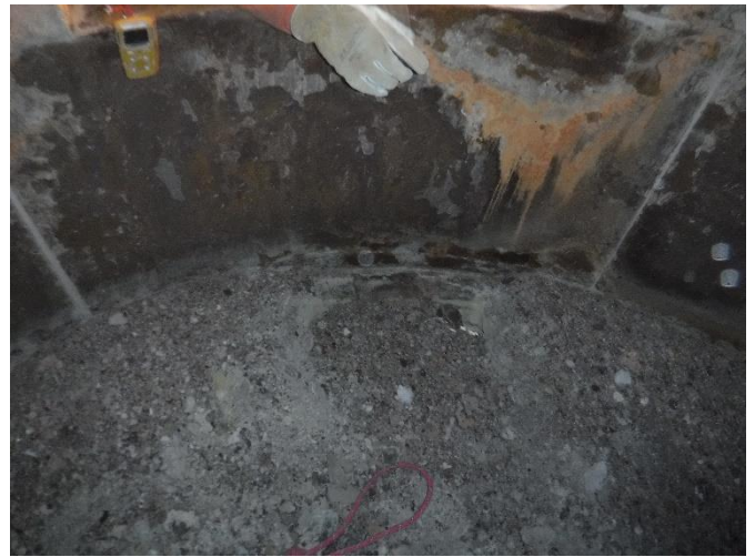
INT 50 – E EL. 0± – View of stack base with debris present
