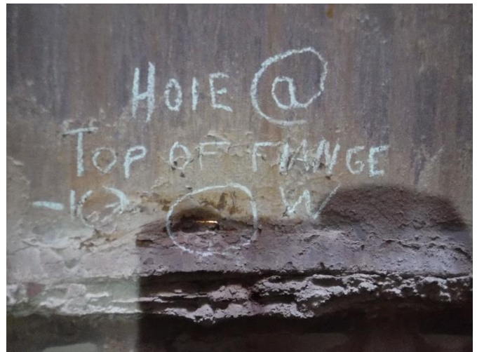
INT 16 – W EL. 170'± – Hole in top of flange
