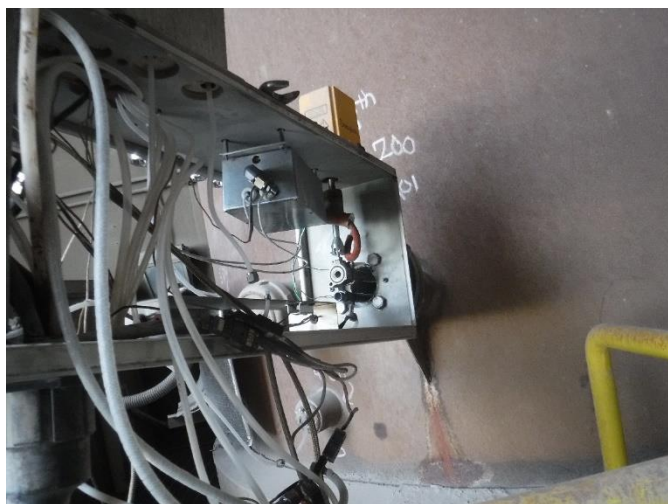
EXT 31 – Instrument missing covers
