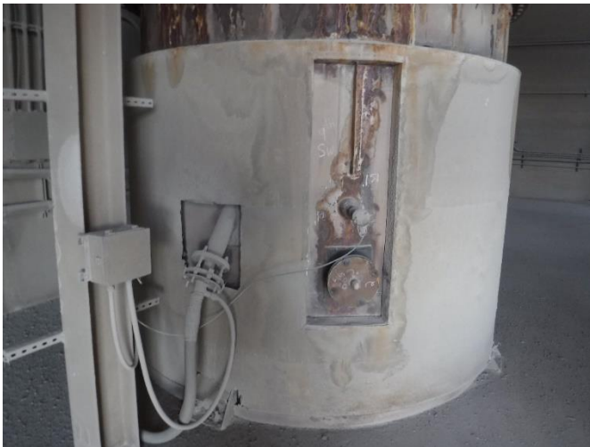
EXT 25 – 9 th floor – oxidized test port and heat shield
