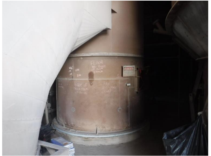
EXT 36 – View of stack base
