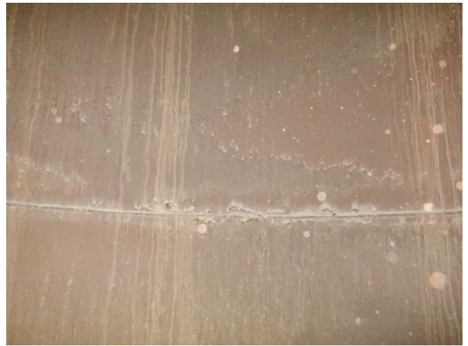
INT 20 – E EL. 160'± – Buildup on flanged joint
