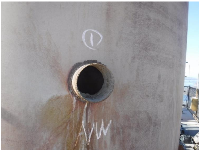
EXT 7 – EL. 200± – Roof port showing signs of corrosion.
