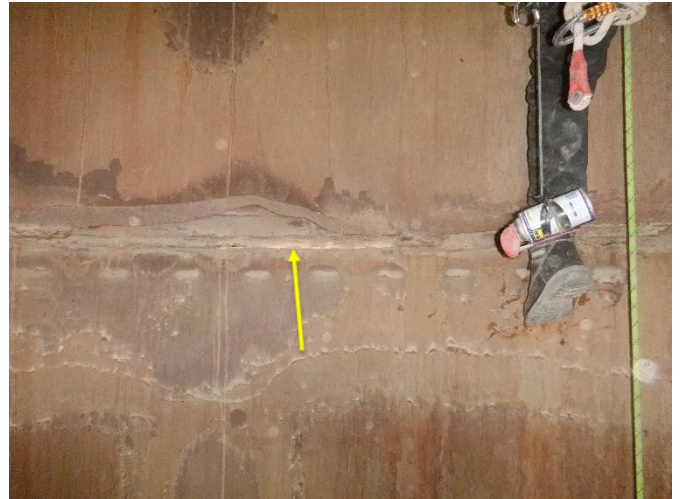
INT 30 – E EL. 127'± – Gap in flanged joint
