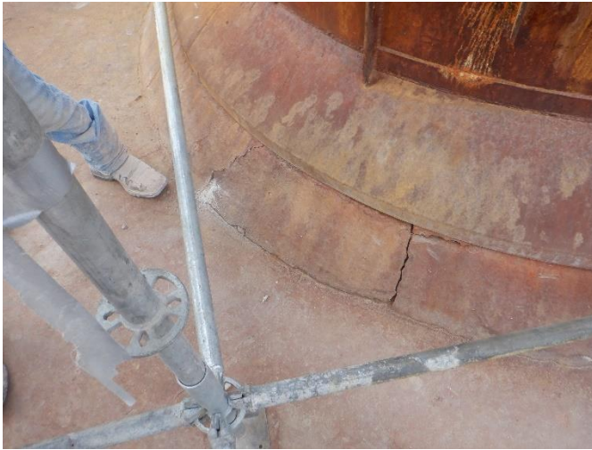
IMG 1 – Typical view of cracked curb before repair
