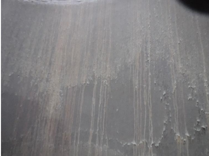
INT 11 – W EL. 170'± – Buildup and stains present on surface of interior
