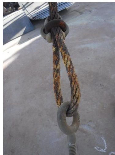
EXT 10 – EL. 200± – Failed coating on guy wire
