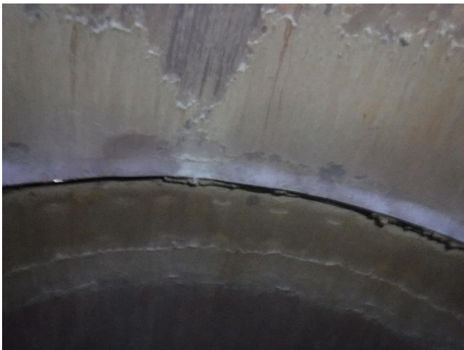
INT 25 – W EL. 130'± – Stack plate appears warped around flanged joint
