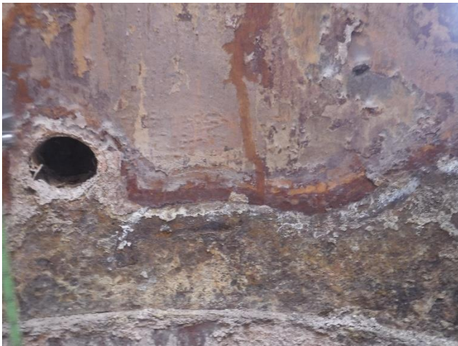
INT 7 – W EL. 190'± – Corrosion and buildup on stack
