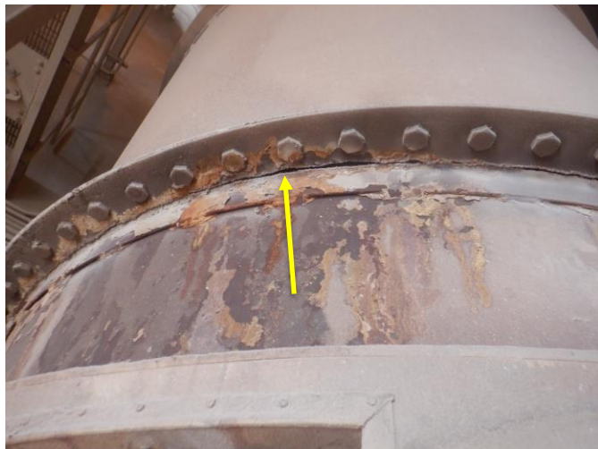
IMG 33 – View of cracked weld on splice flanged
