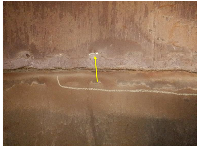
INT 14 – E EL. 170'± – Holes and gap near flanged joint
