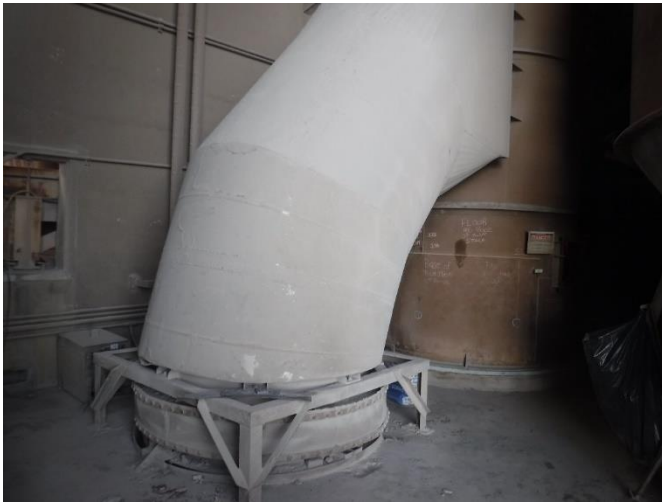
EXT 41 – 6 th Floor – Breeching duct and support frame
