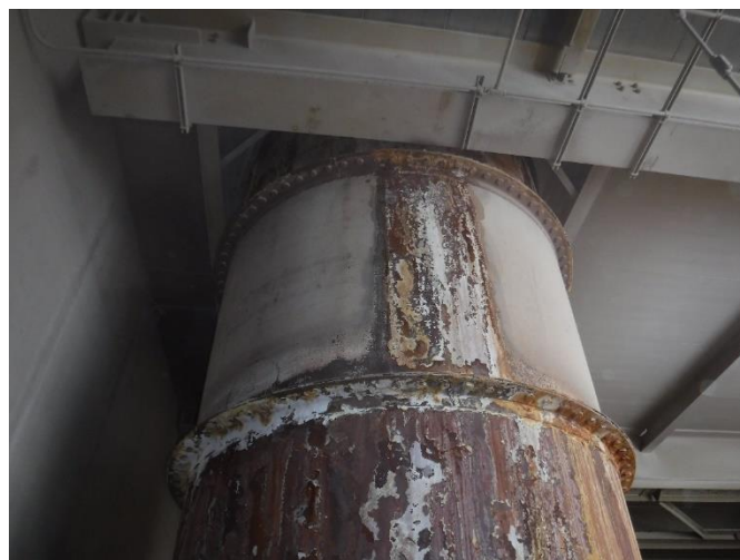
EXT 22 – 10 th floor – Oxidation and stains from leakage
