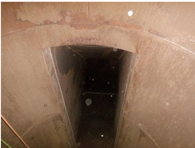
INT 45 – E EL. 40± – Breeching duct opening
