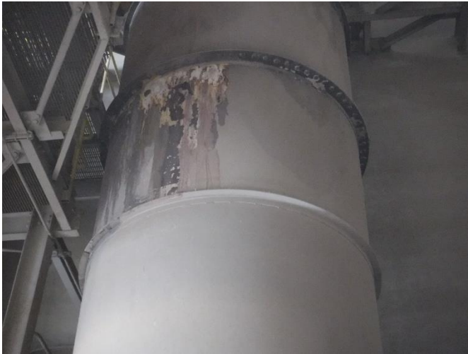
EXT 23 – 9 th floor – showing stains from leakage
