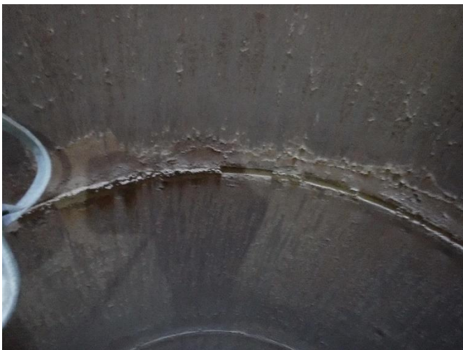
INT 21 – W EL. 150'± – Buildup on flanged joint
