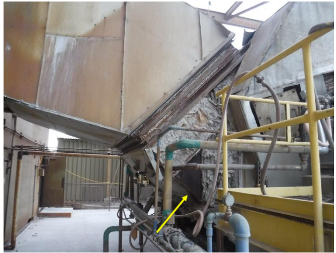
EXT 44 – Breeching showing oxidation and torn cladding
