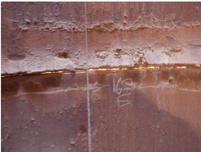
INT 15 – E EL. 170'± – Gap in flanged joint
