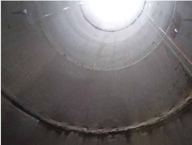
INT 23 – W EL. 140'± – Upward view of stack interior; flanged joint exhibiting buildup
