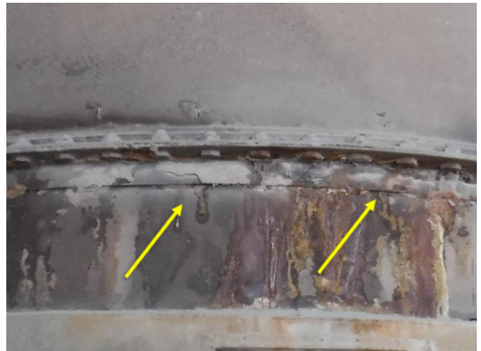
EXT 26 – 9 th Floor – Cracked weld on splice flanged before repairs
