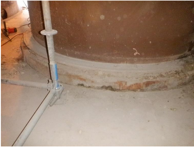
IMG 13 – The base before repair process
