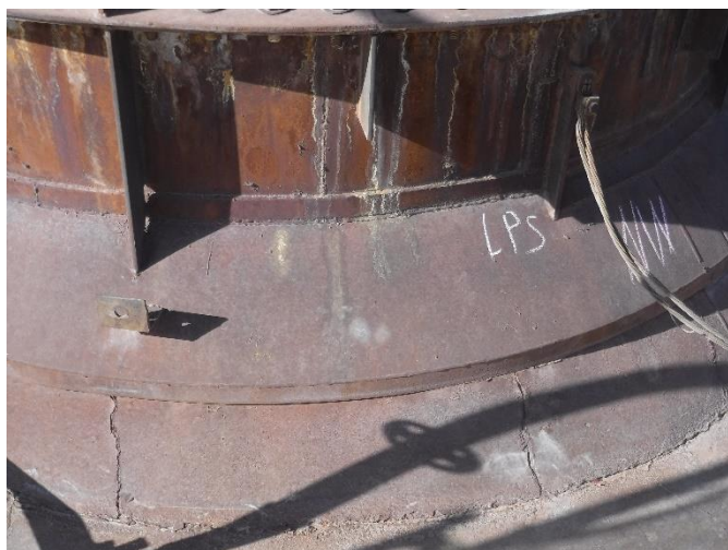
EXT 19 – Roof – Cracks present on curb before repairs
