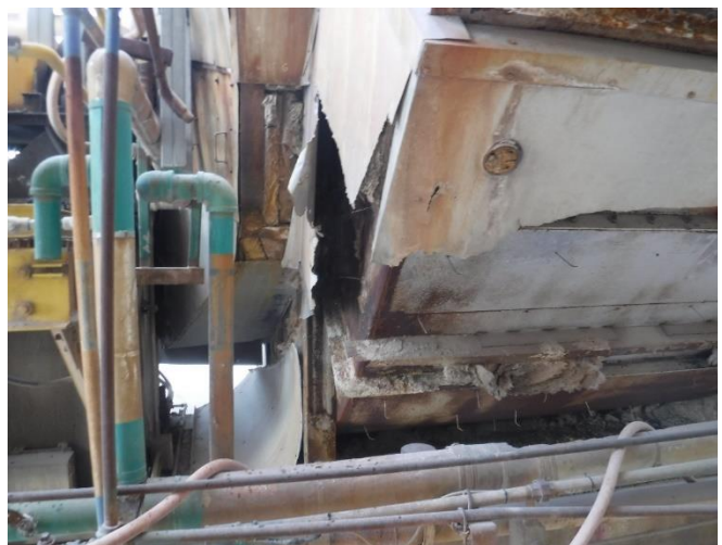
EXT 46 – Breeching showing oxidation and torn cladding
