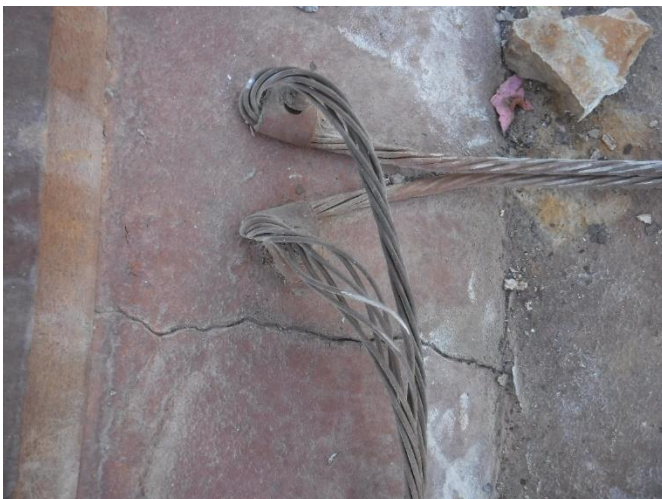
EXT 15 – Frayed LPS conductor, crack on curb. Debris present on rooftop
