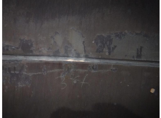
INT 42 – W EL. 60± – Gap in joint
