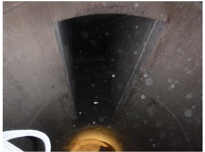
INT 44 – E EL. 40± – Breeching duct opening
