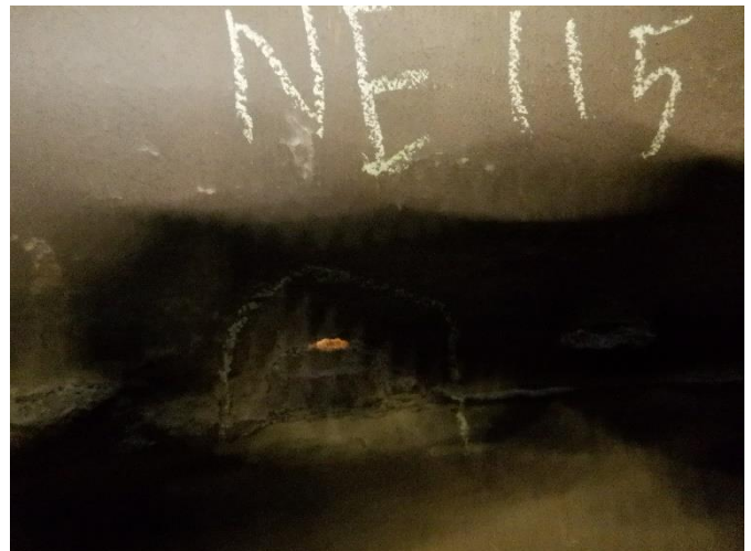
INT 34 –W EL. 115'± – Hole near joint
