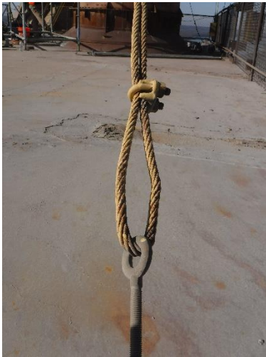
EXT 11 – EL. 200± – Failed coating on guy wire
