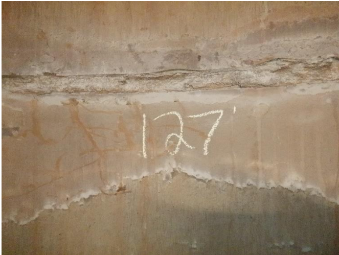
INT 29 – E EL. 127'± – Flanged joint exhibiting buildup
