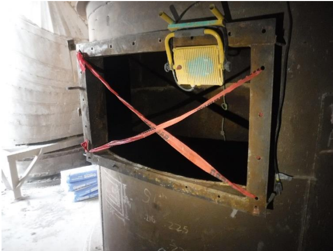
EXT 37 – Access point
