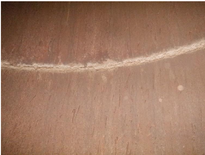
INT 43 – E EL. 40± – View of buildup at flanged joint
