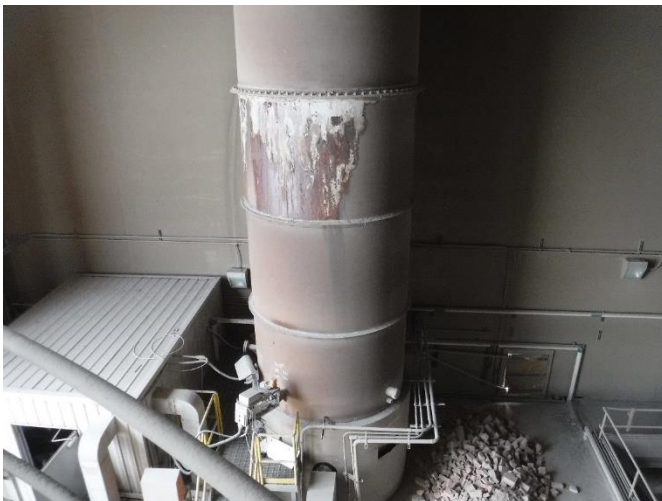
EXT 27 – 8 th Floor – Leakage stains through flanged joint
