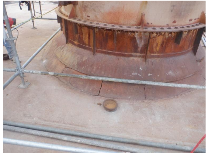
IMG 2 – Typical view of cracked curb before repair
