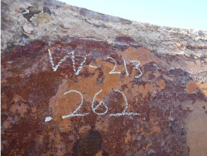
INT 1 – W EL. 213'± – Top of the stack, buildup heavy oxidation present
