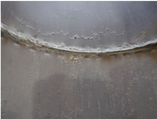
INT 19 – W EL. 160'± – Buildup/ warped flanged joint
