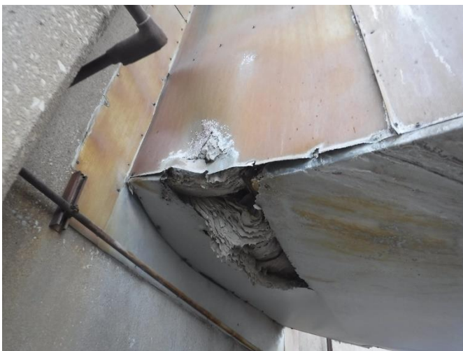
EXT 45 – Breeching duct with torn cladding on the underside
