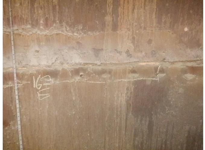
INT 12 – E EL. 170'± – Gap in flanged joint
