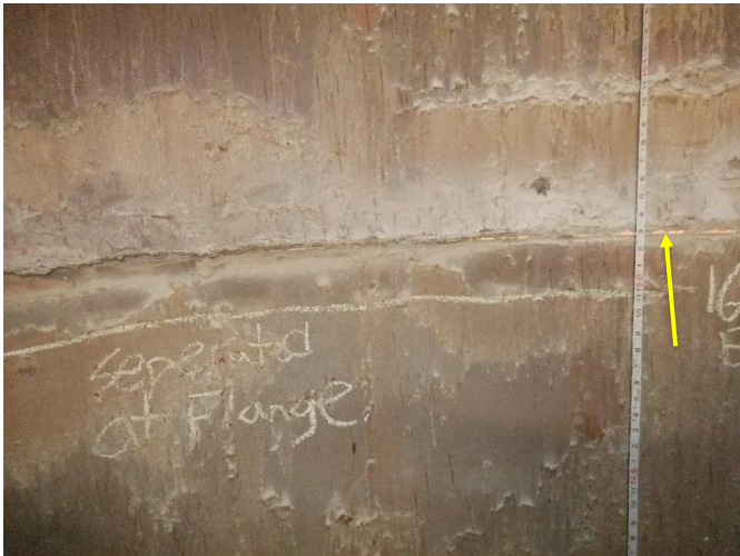
INT 13 – E EL. 170'± – Splice separated at flange
