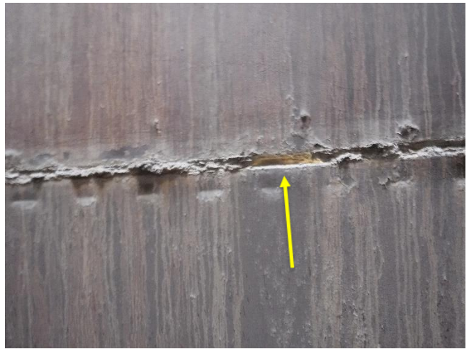
INT 8 – W EL. 180'± – Gap in flanged joint
