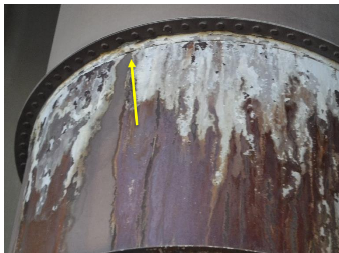
EXT 20 – 10 th Floor – Roof penetration, leakage through flanged joint. Gaps are present in splice flanged before repairs
