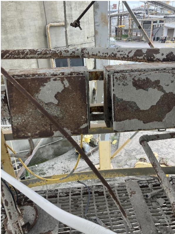
EXT 39 – Heavy oxidation on electrical boxes
