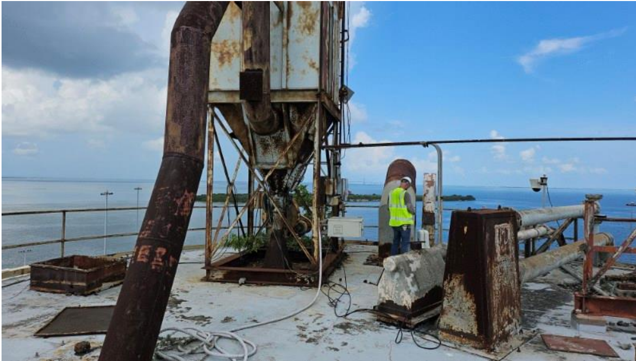
EXT 12 – Silo instruments and fixtures are heavily corroded
