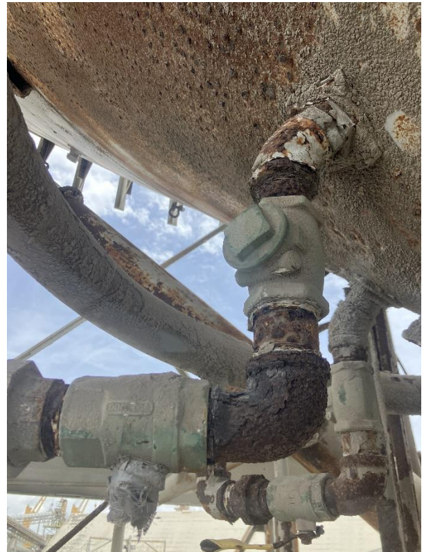
EXT 40 – Corroded pipes
