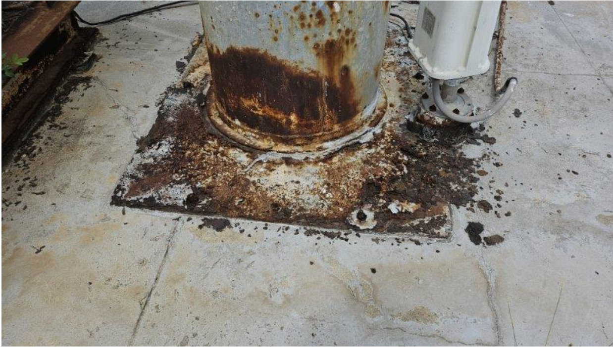
EXT 16 – Pipe base plate is corroded which could lead to falling object hazard
