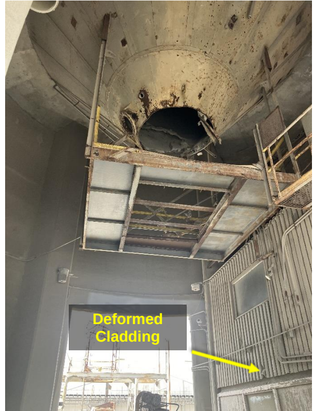
EXT 10 – Hopper and surrounding members suffer oxidation, cladding deformed
