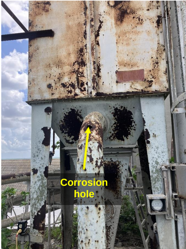
EXT 30 – Corrosion hole in present in hopper
