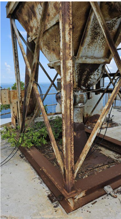
EXT 20 – Hopper suffers heavy oxidation and onset corrosion
