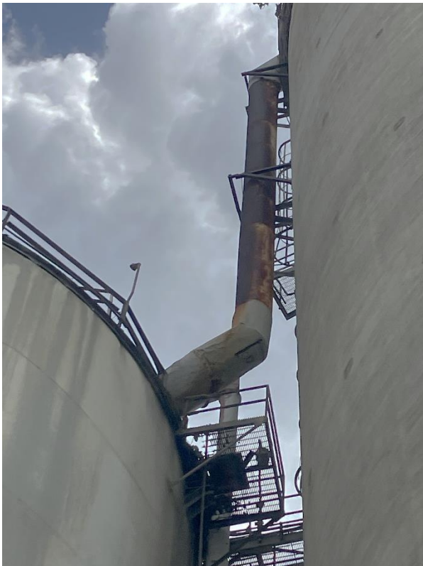
EXT 3 – Heavily oxidized duct
