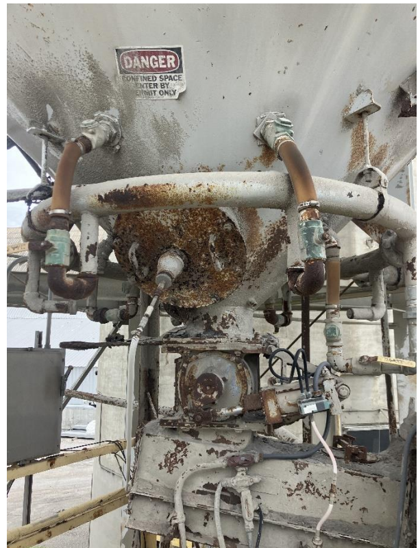
EXT 36 – Hopper components are corroded
