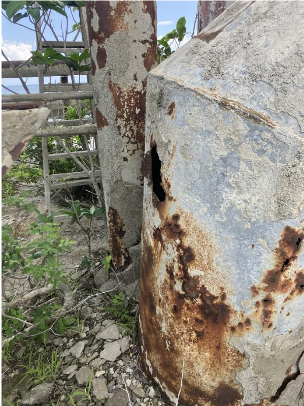
EXT 22 – Attachment points is corroding away
