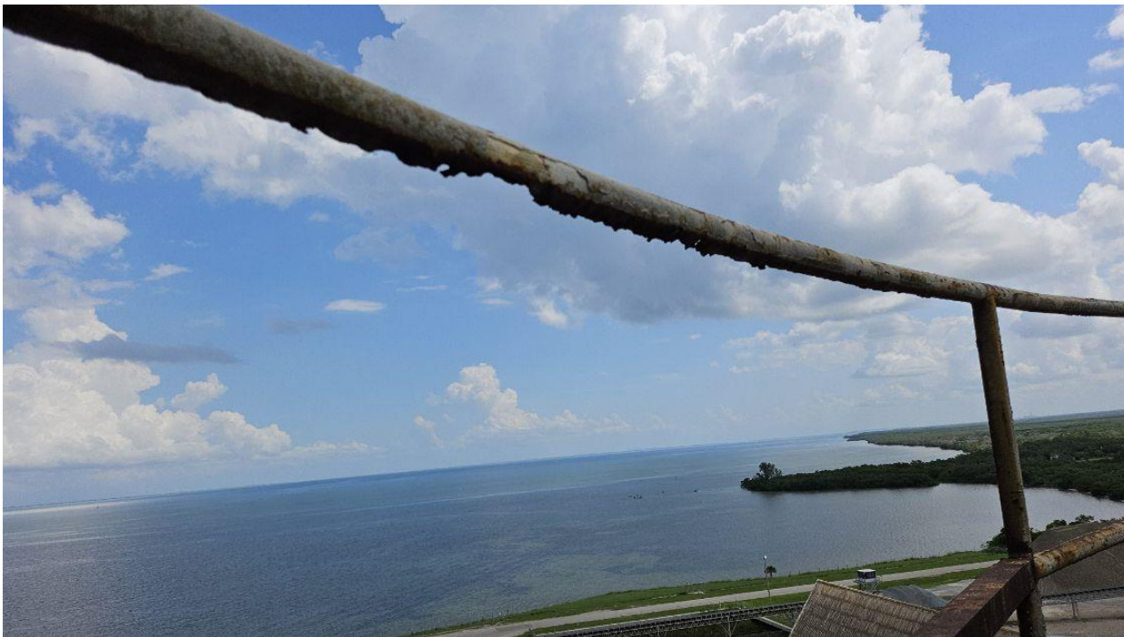
EXT 17 – The guardrail and its members suffer from heavy oxidation and corrosion
