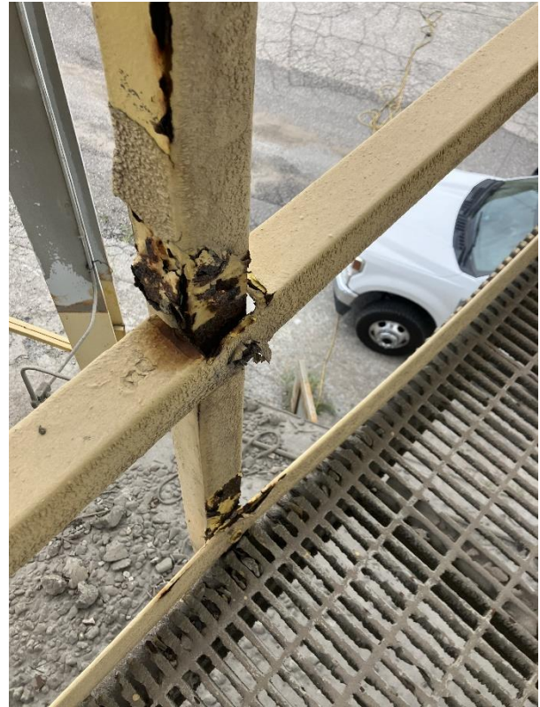
EXT 42 – Post is rusting through
