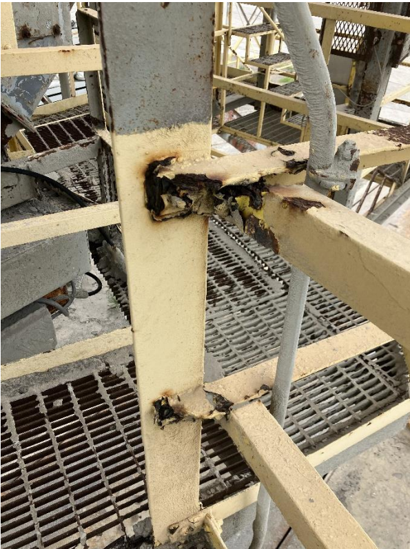
EXT 43 – Heavy oxidation on guardrail
