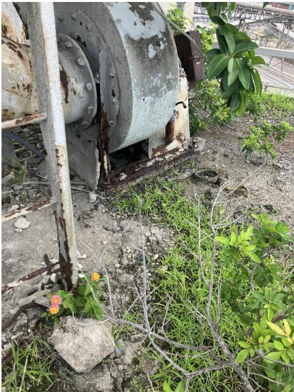
EXT 24 – Corroding components; ladder component corroding
