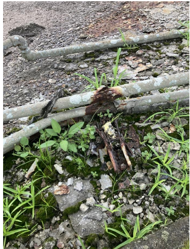
EXT 29 – Conduit components show heavy oxidation and corrosion
