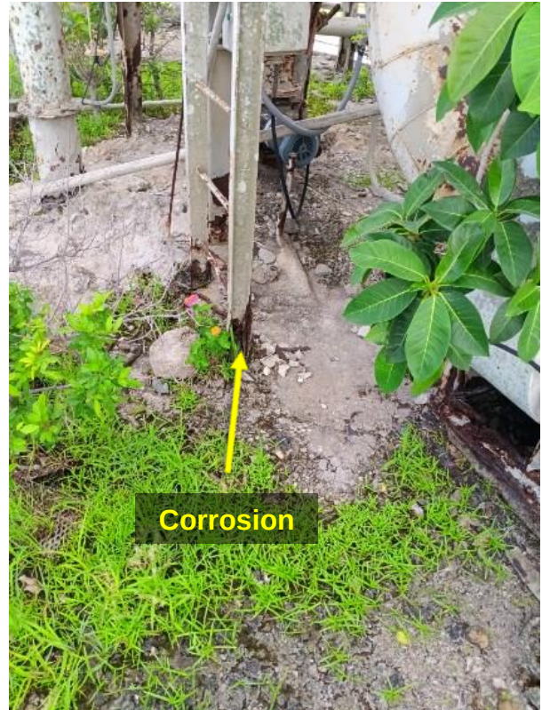
EXT 31 – Ladder base has started to corrode
