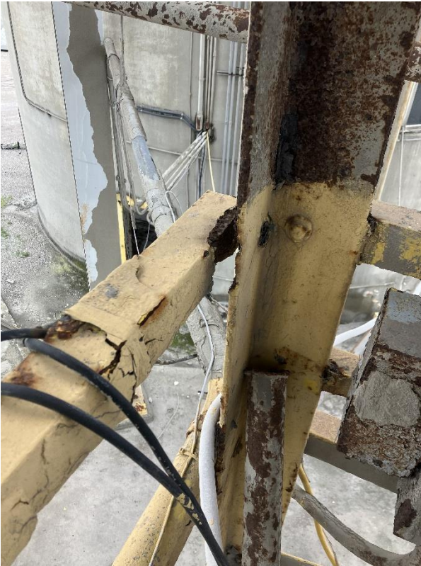
EXT 41 – Guardrail and components are corroding
