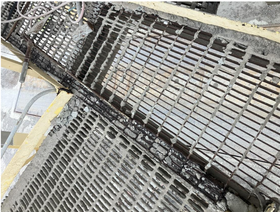
EXT 46– Heavy buildup and oxidation on grating
