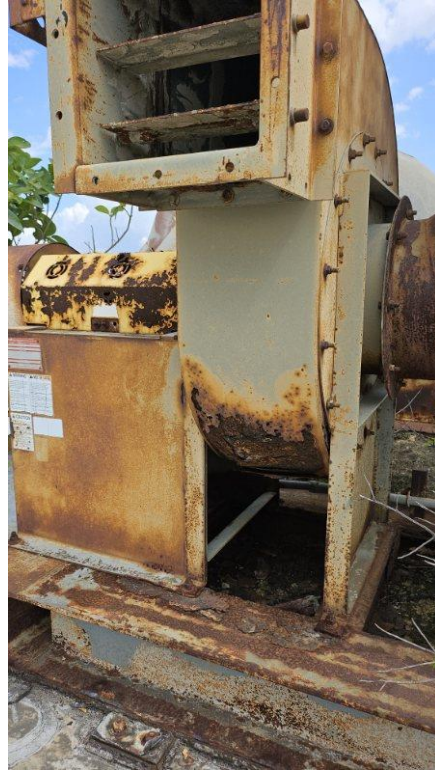
EXT 19 – Vent system is corroded
