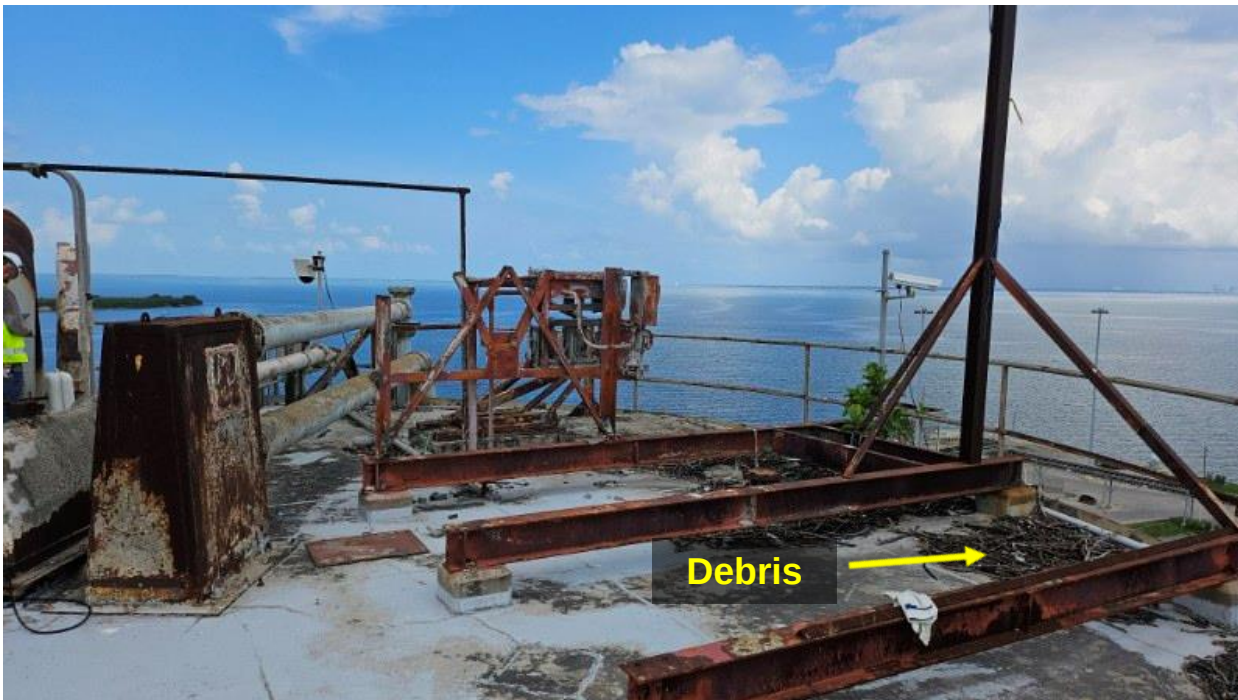
EXT 13 – Silo instruments and fixtures are heavily corroded; piles of debris present on rooftop
