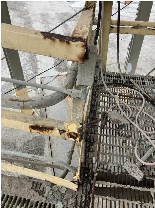
EXT 35 – Guardrails are heavily corroded
