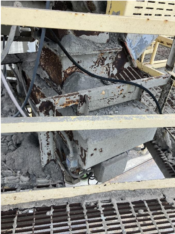
EXT 37 – Base of structure members are corroding
