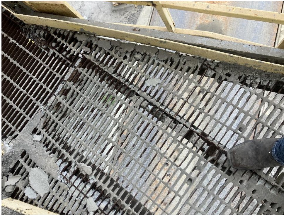
EXT 45 – Heavy buildup and oxidation on grating
