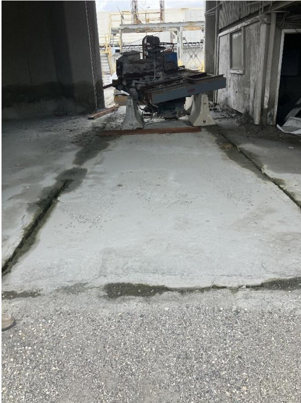
EXT 9 – Corroded loadout scale & with heavy buildup present
