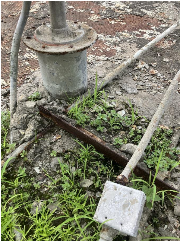
EXT 28 – Conduit components show heavy oxidation and corrosion
