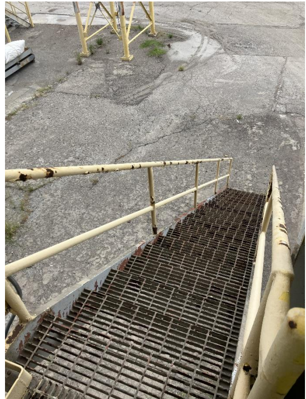
EXT 44 – Stairs and guardrail exhibit heavy oxidation
