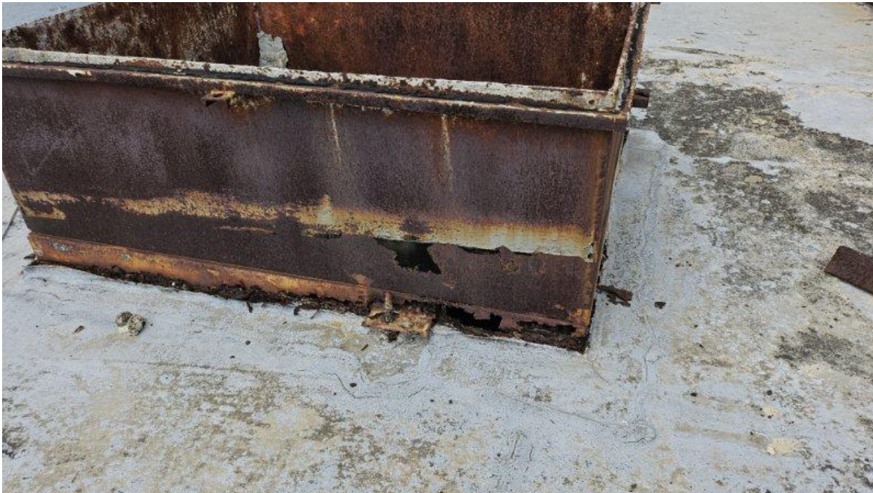
EXT 15 – Closeup on corrosion hole
