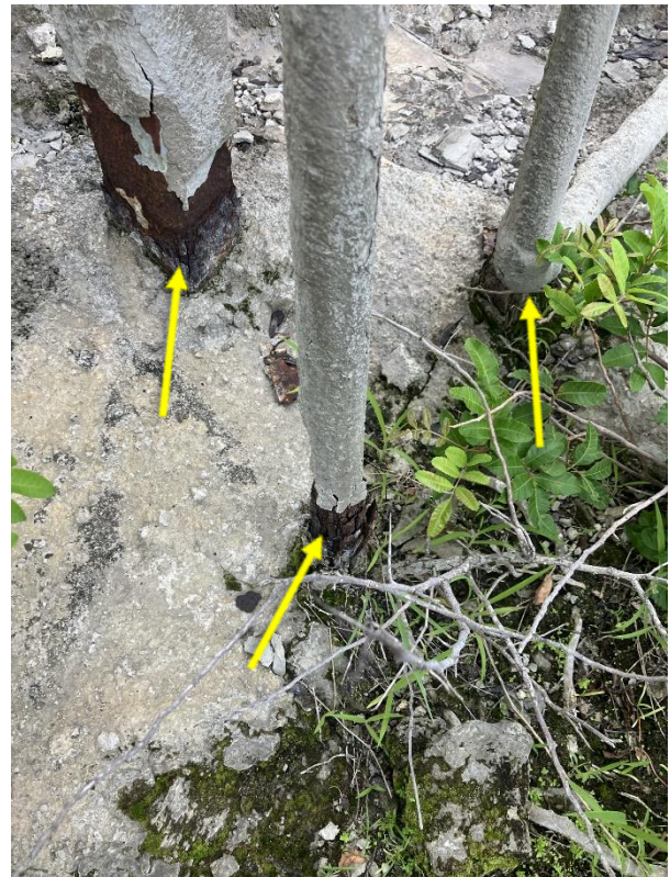
EXT 25 – Post base components have corroded; hazardous
