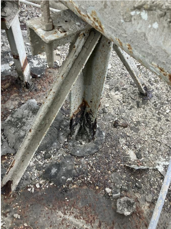
EXT 26 – Base of structure members are corroding
