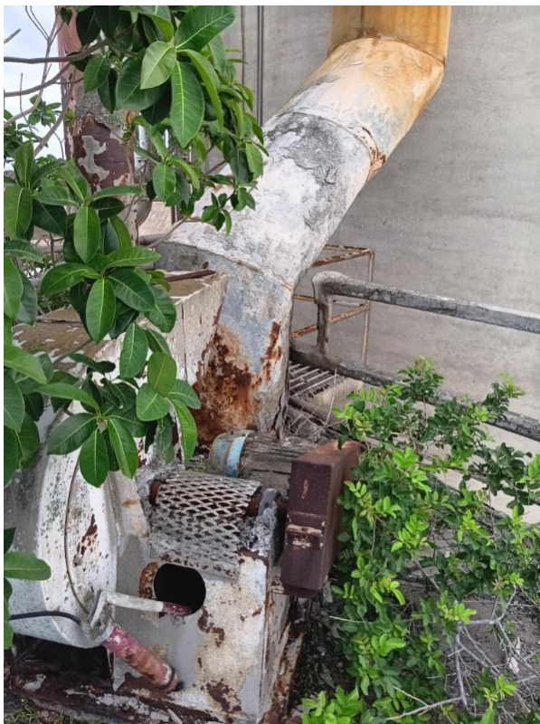
EXT 32 – Heavy corrosion on components
