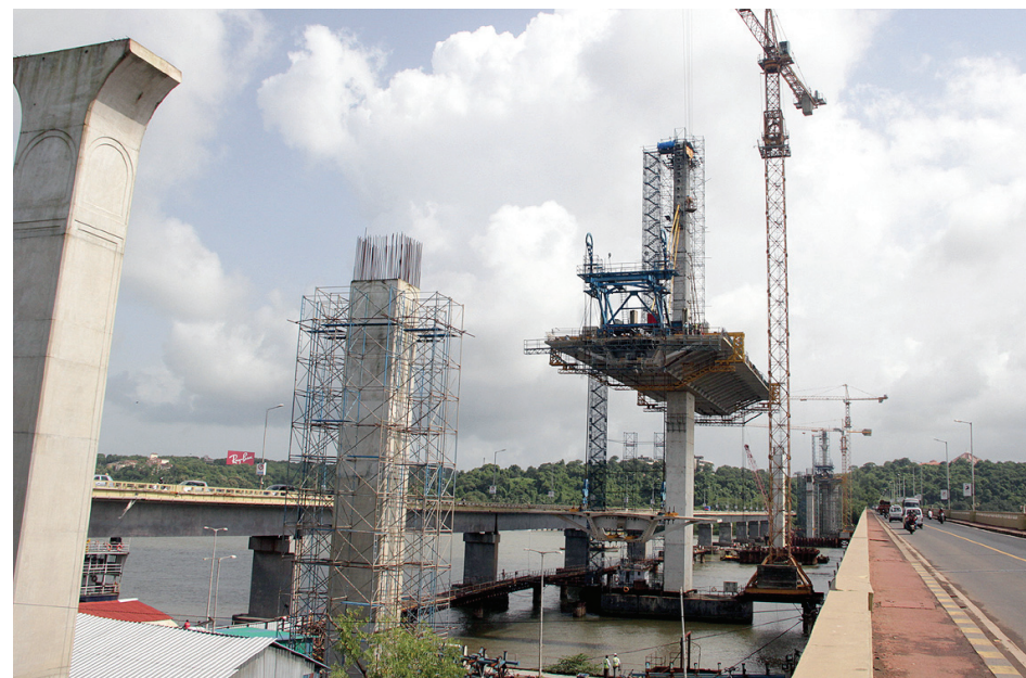
The work on the construction of third Mandovi bridge has been going on at the highest level of activity.
