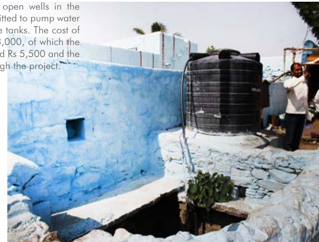
Fitting each well with a motor made it much easier to pump water into the storage tanks.
