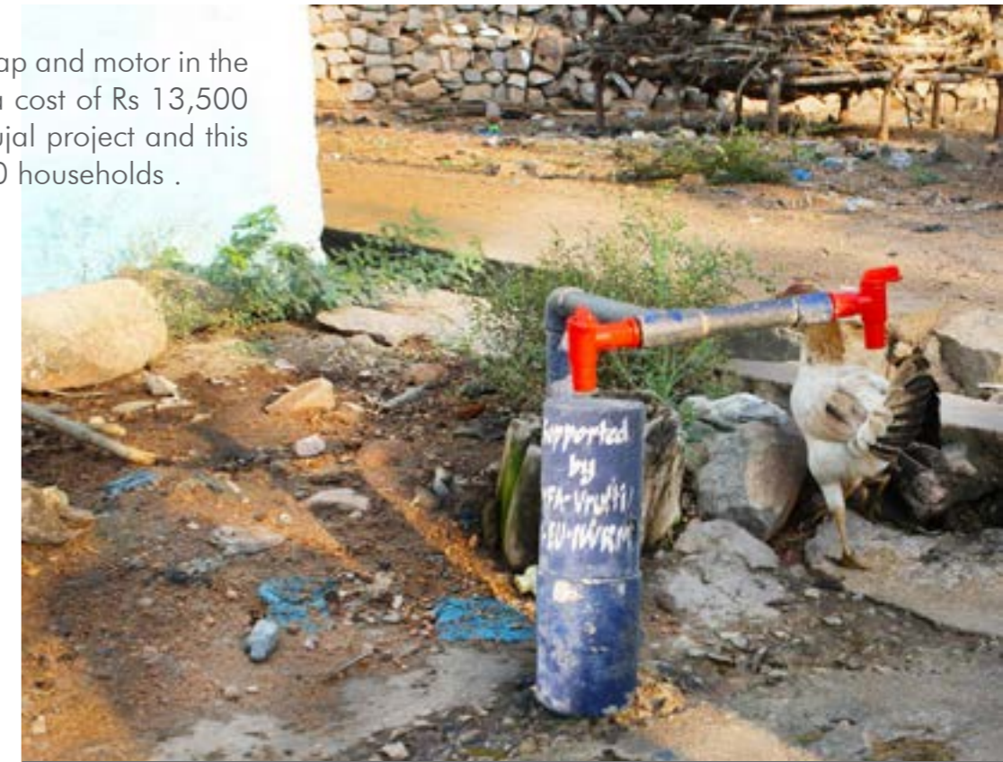
The new tap connections have brought water from the overhead tank closer to people's homes.
