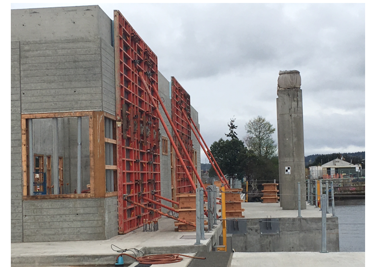
The walls of the passenger building are up on the Mukilteo waterfront along with supports for the overhead passenger walkway.
