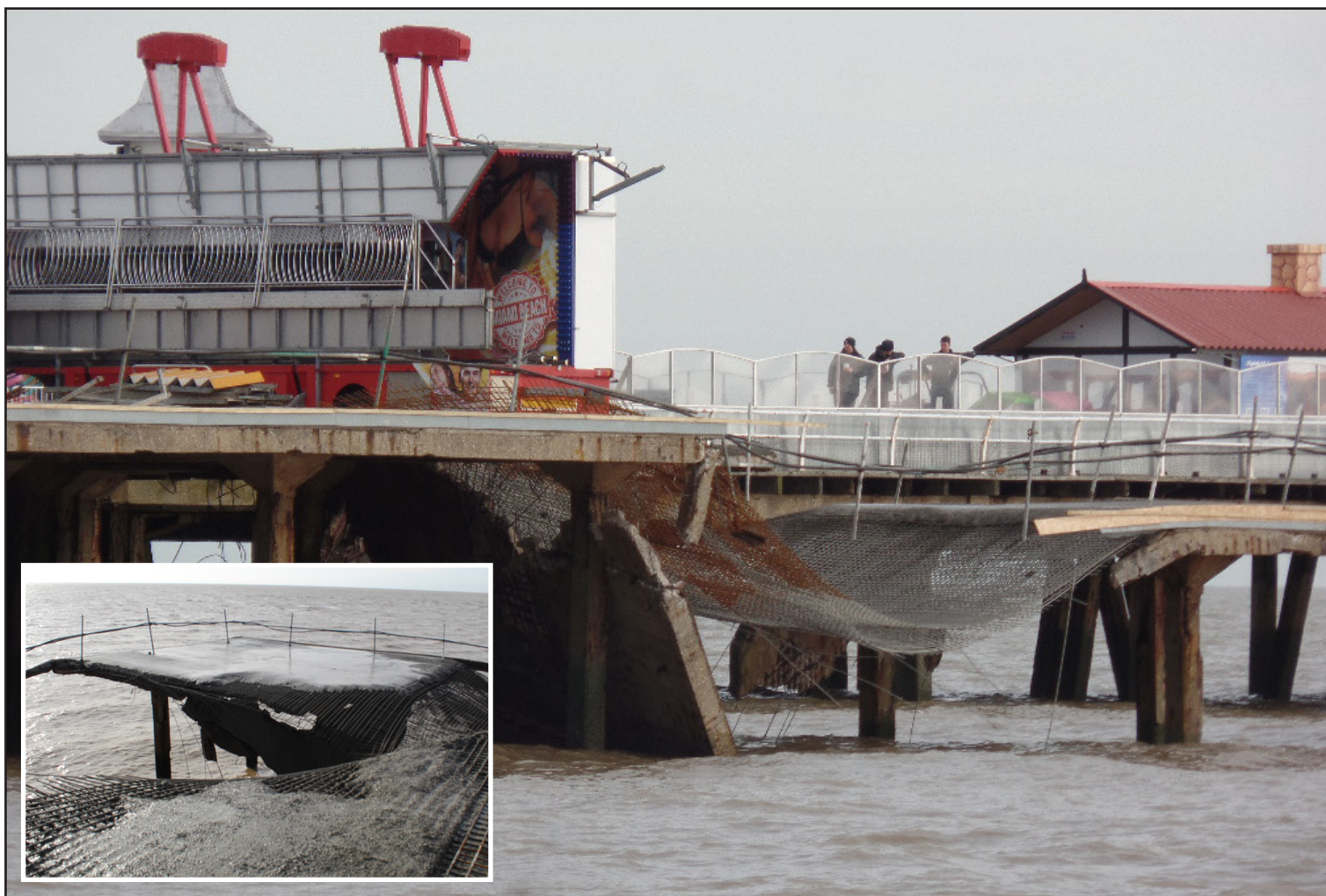
■ Collapse - a section of Clacton Pier plunged into the North Sea and (inset) the hole left on the deck after the incident
