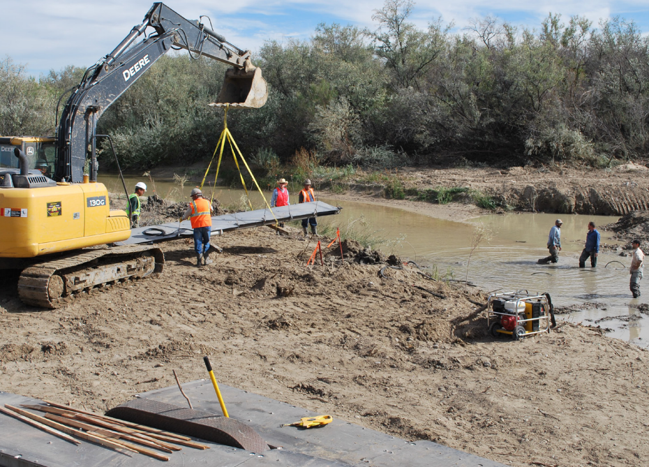
Installation of a flat-plate, pass-by antenna to track tagged fish in a shallow channel of the San Juan River. © Mark McKinstry
