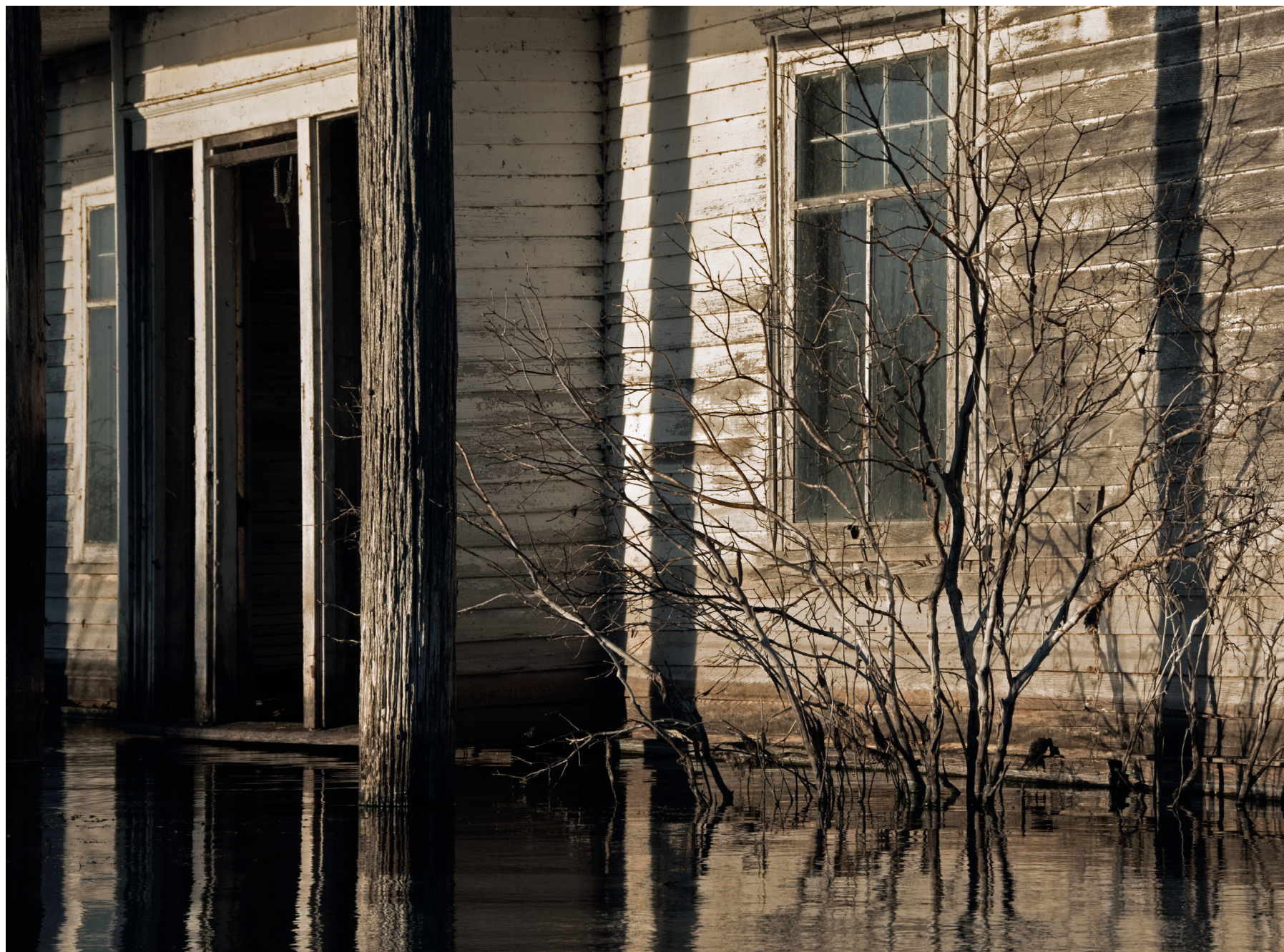
ABOVE AND OPPOSITE Johnson recalls his frame of mind on the day he rowed past this century-old house, submerged for 15 years now: "I thought about the generations that grew up here and imagined how hard it must have been to have water slowly take away their heritage." While shooting, the photographer encountered partially sunken plows, augers, and farm trucks—hazardous debris to area boaters and ghosts of livelihoods lost.
