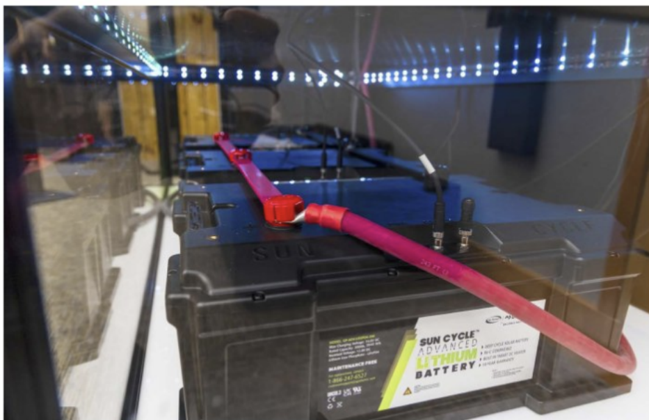
Go Power's PowerBoard System has three batteries to provide energy for the 48-volt system.
