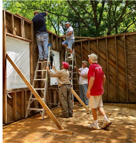
(Above) With the help of a dedicated work crew, rafters have now been added to the Schoolhouse. Photo by Gary Barton.
