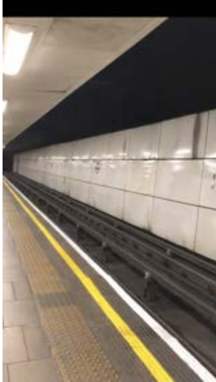
Figure 20 - A white brick wall with no advertisements at Mile End station (Photo taken by the researcher).
