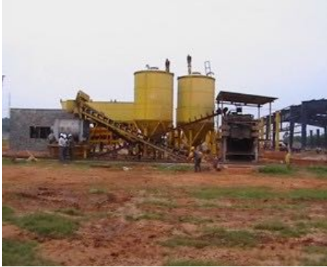
Concrete Weight Coating Plant
