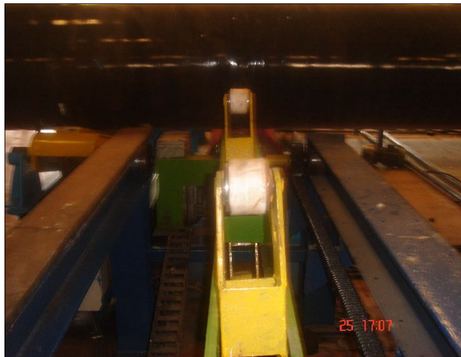
Pipe Rolling System
